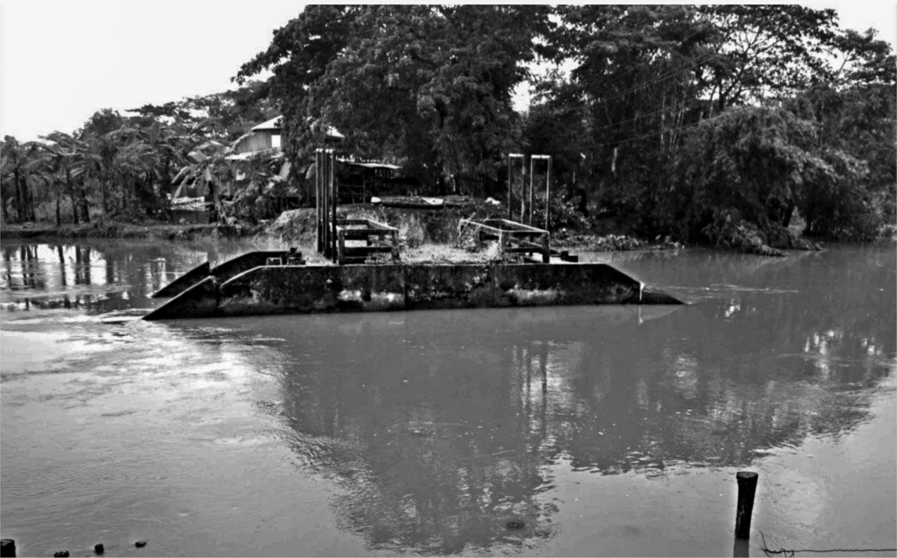
The collapsed dyke beside the useless sluice gate on Bauria canal in Patuakhali's Galachipa upazila remains without repair since it was washed away in June, 2015. The photo was taken recently. PHOTO: SOHRAB HOSSAIN
