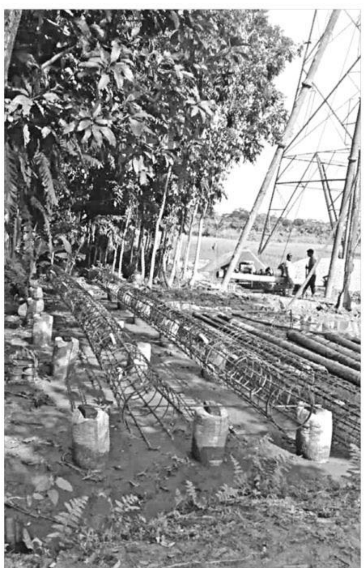
Construction work underway on the land, being carried out by Rural Electrification Board.
