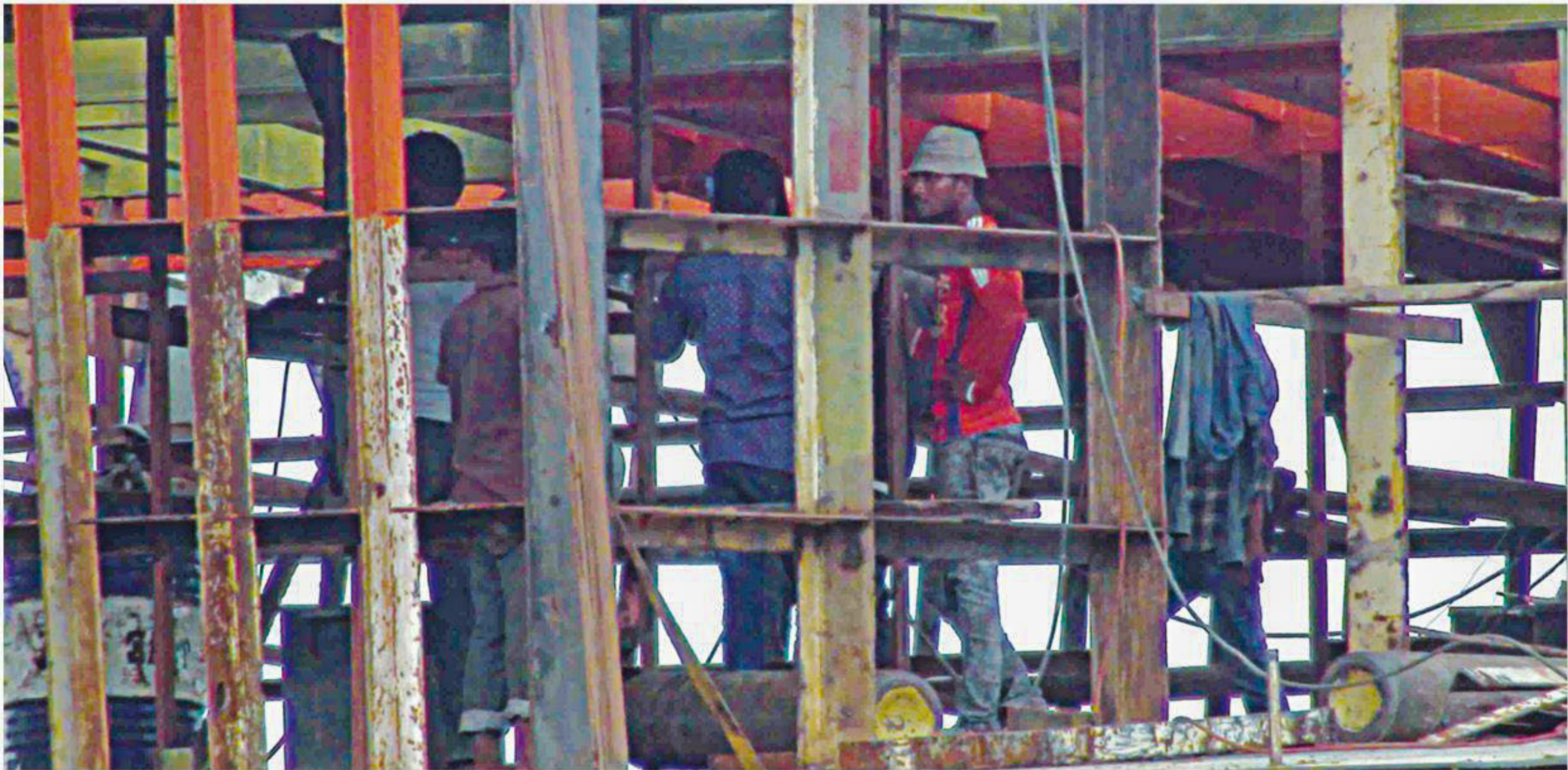
Workers building a ship without using any safety equipment at a dockyard near Nesarabad Bus Terminal under Nesarabad upazila of Pirojpur. The photo was taken recently.
