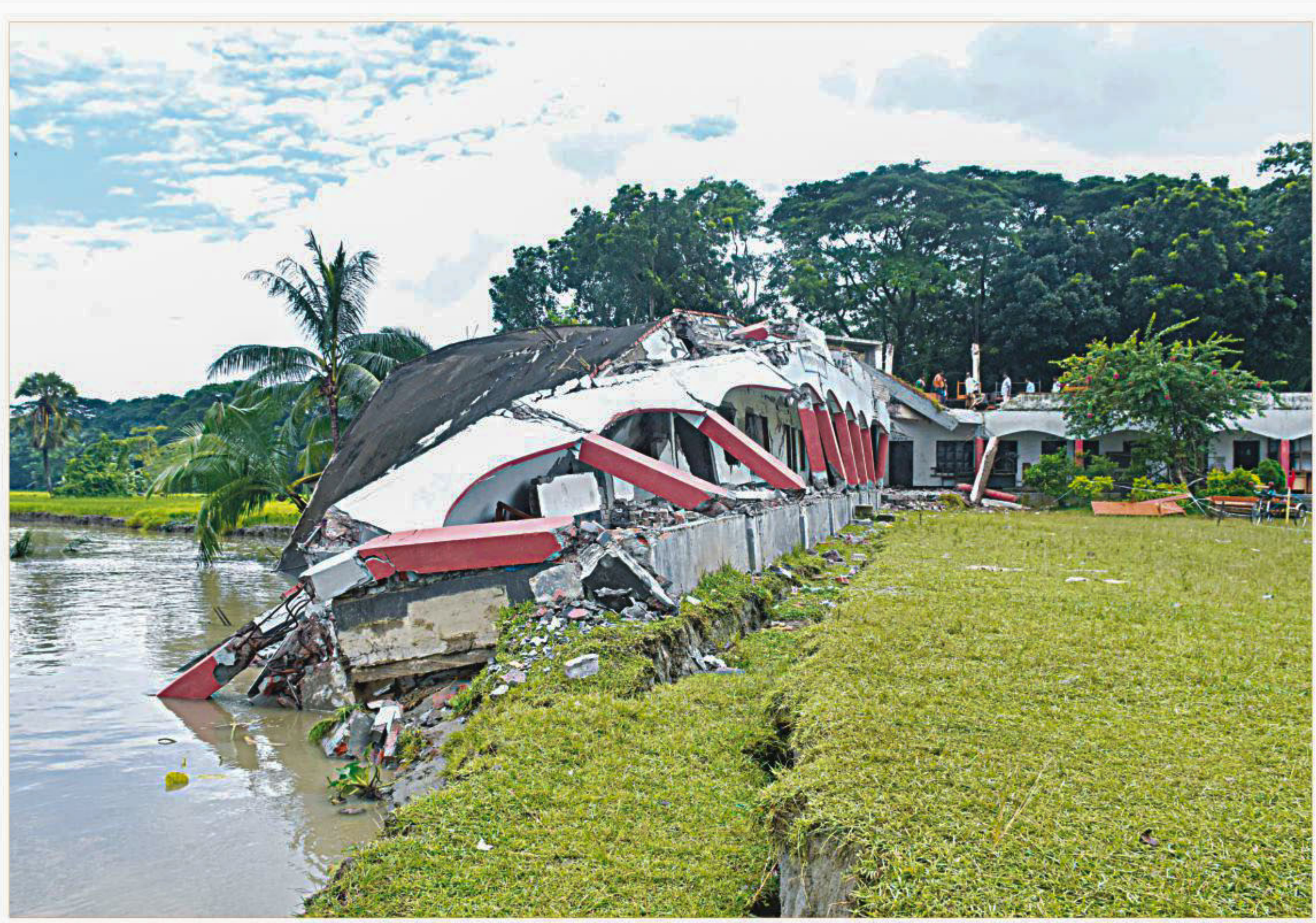
The Sugandha river devours Syed Rashida Mosharrar Academy, a high school near Bir Sreshtho Mohiuddin Jahangir Bridge in Barisal's Babuganj upazila yesterday. Erosion of the river bank has taken a serious turn in last two days as over 10 houses and a vast area of farmland have been engulfed. PHOTO: STAR
