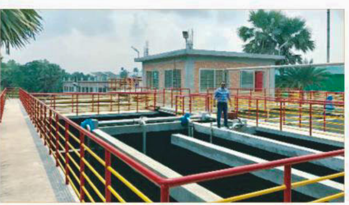
The effluent treatment plant of Mayble & Frank Ltd in Bhaluka, Mymensingh.
