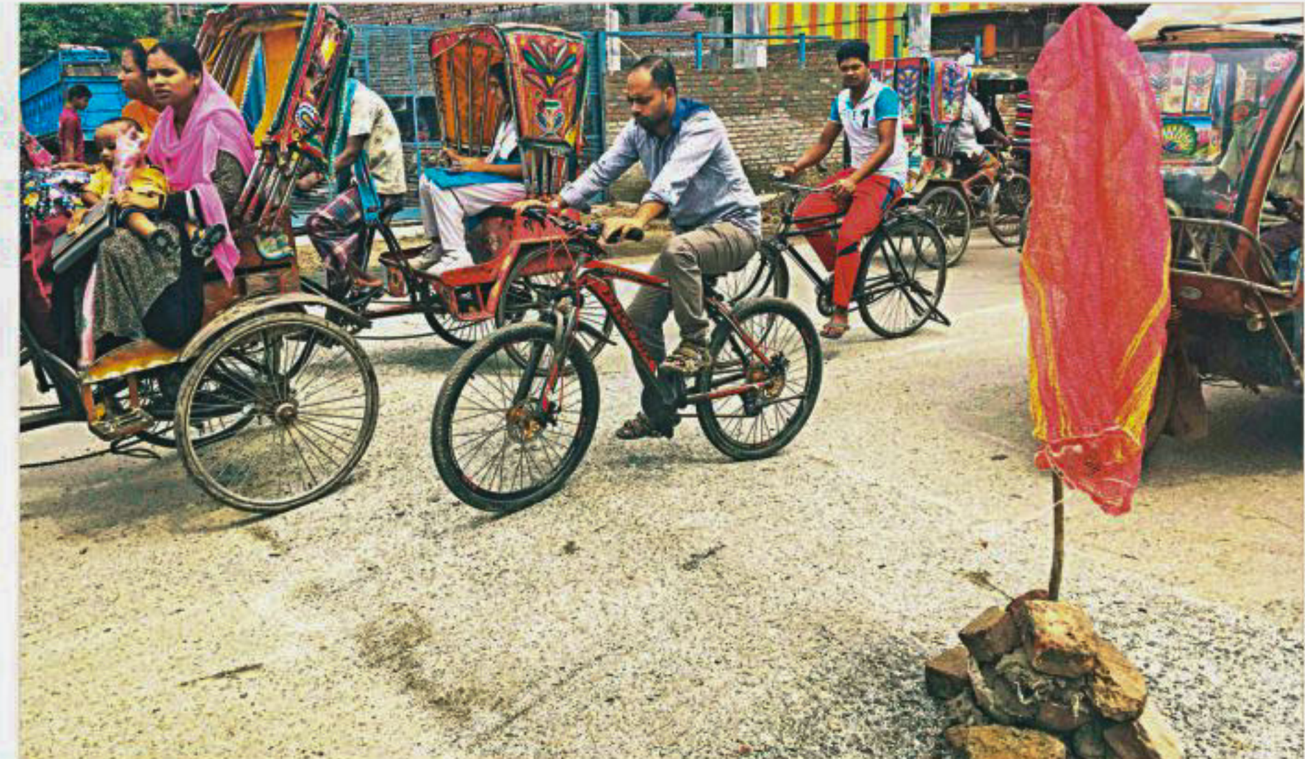
An unauthorised speed breaker in front of Rajshahi Education Board Government Model School and College in Shalbagan area of Rajshahi city. The Rajshahi City Corporation built it last week in violation of a road safety action plan following directives of the government.
