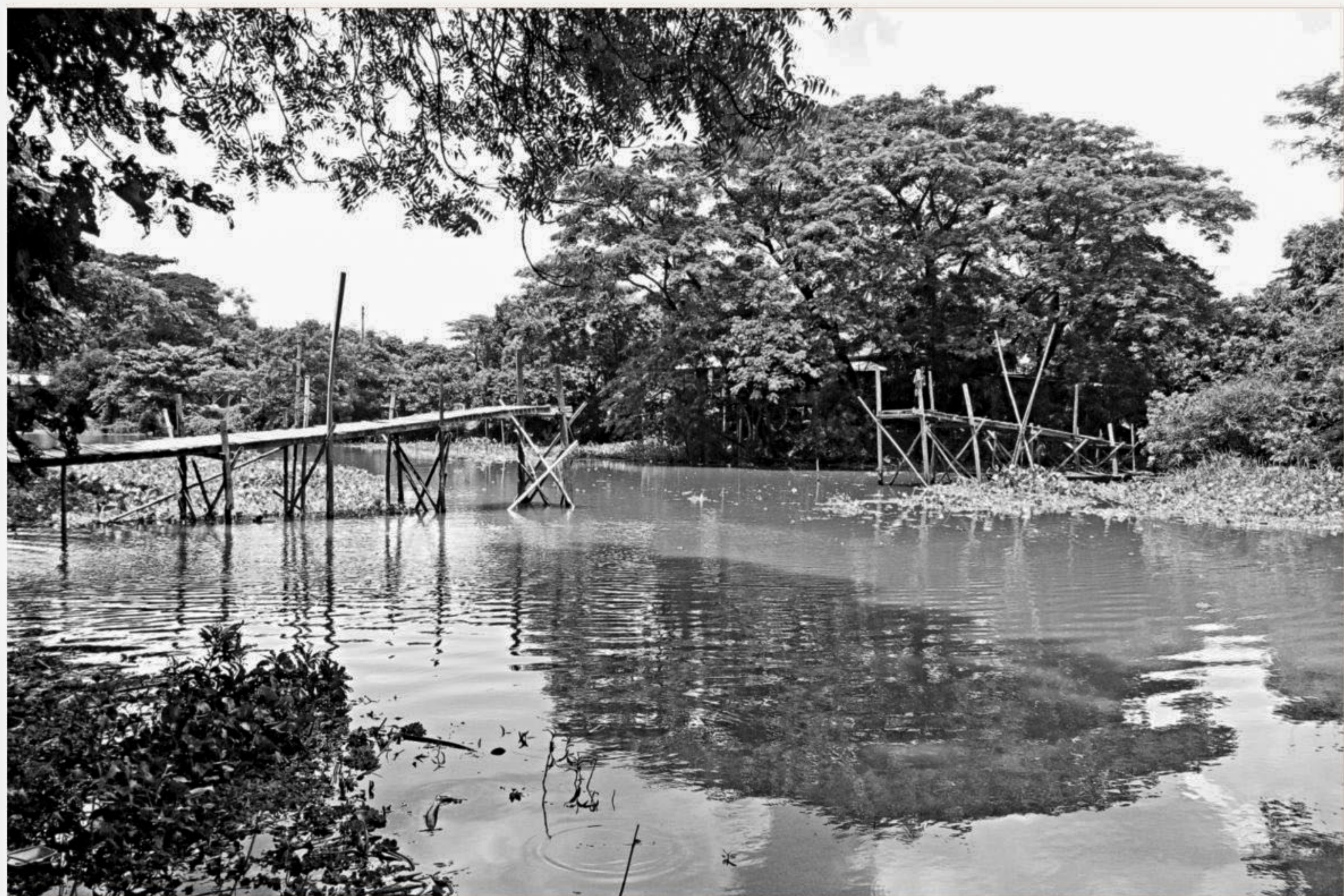
This wooden bridge on Syedpur canal near Bhairab Bari launch terminal in Shologhar union under Sreenagar upazila of Munshiganj lies useless for a couple of months during the ongoing rainy season as a syndicate of sand traders removed its middle part to enable movement of sand carrying boats.
