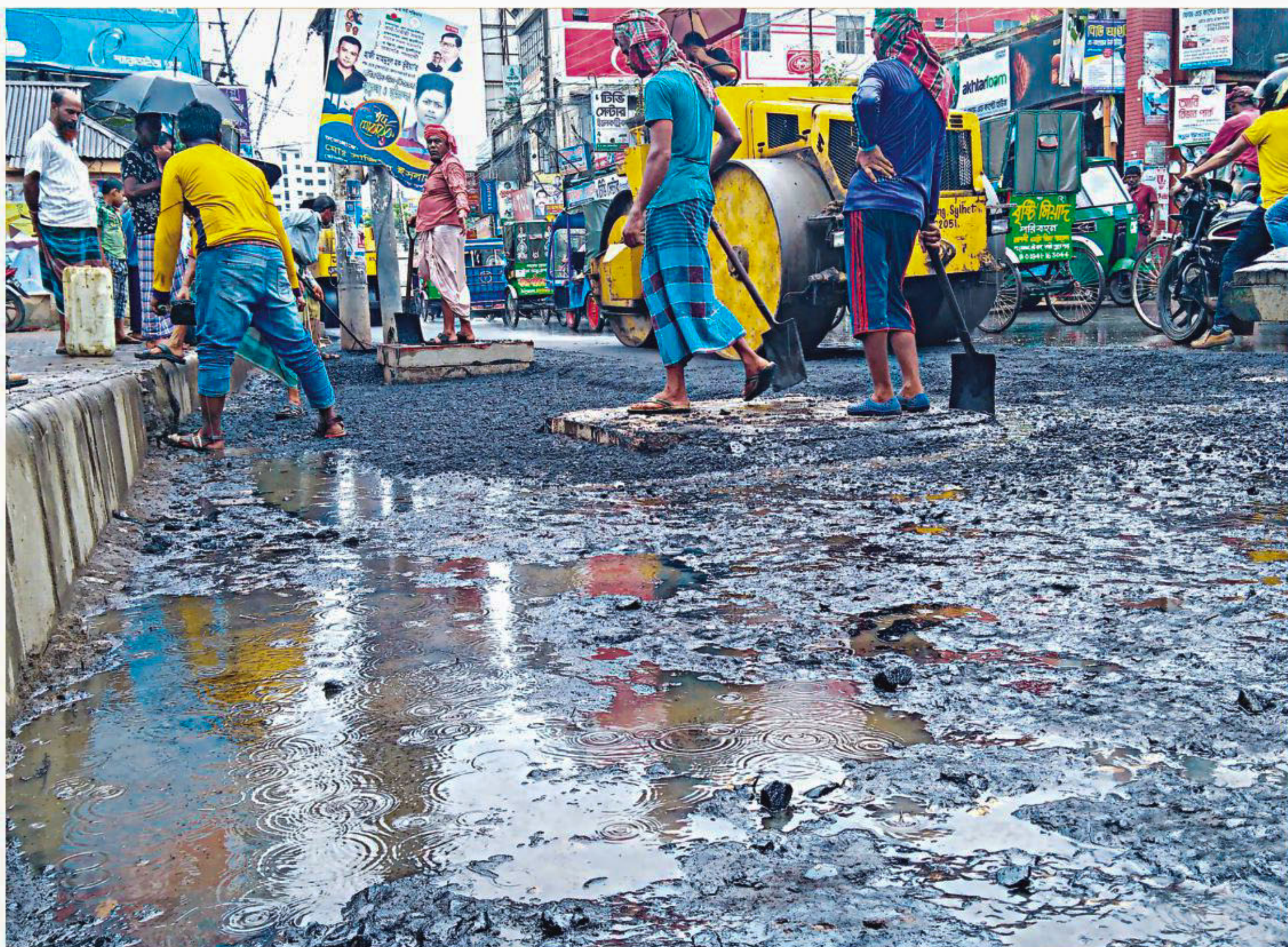
Workers resurface the thoroughfare of Brahmanbaria town, TA Road, amid rain yesterday afternoon.
