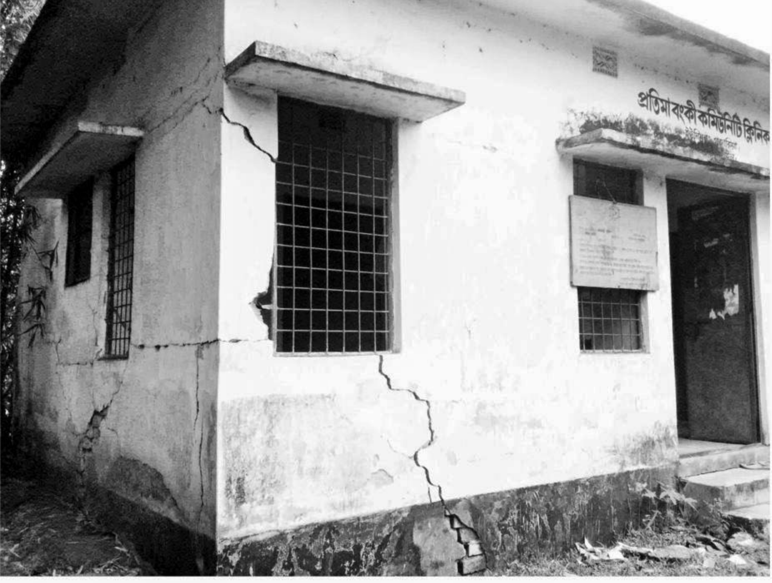
Cracks have developed on the walls of Protima Bonki Community Clinic in Sakhipur upazila of Tangail, posing great risk to the patients and workers.
