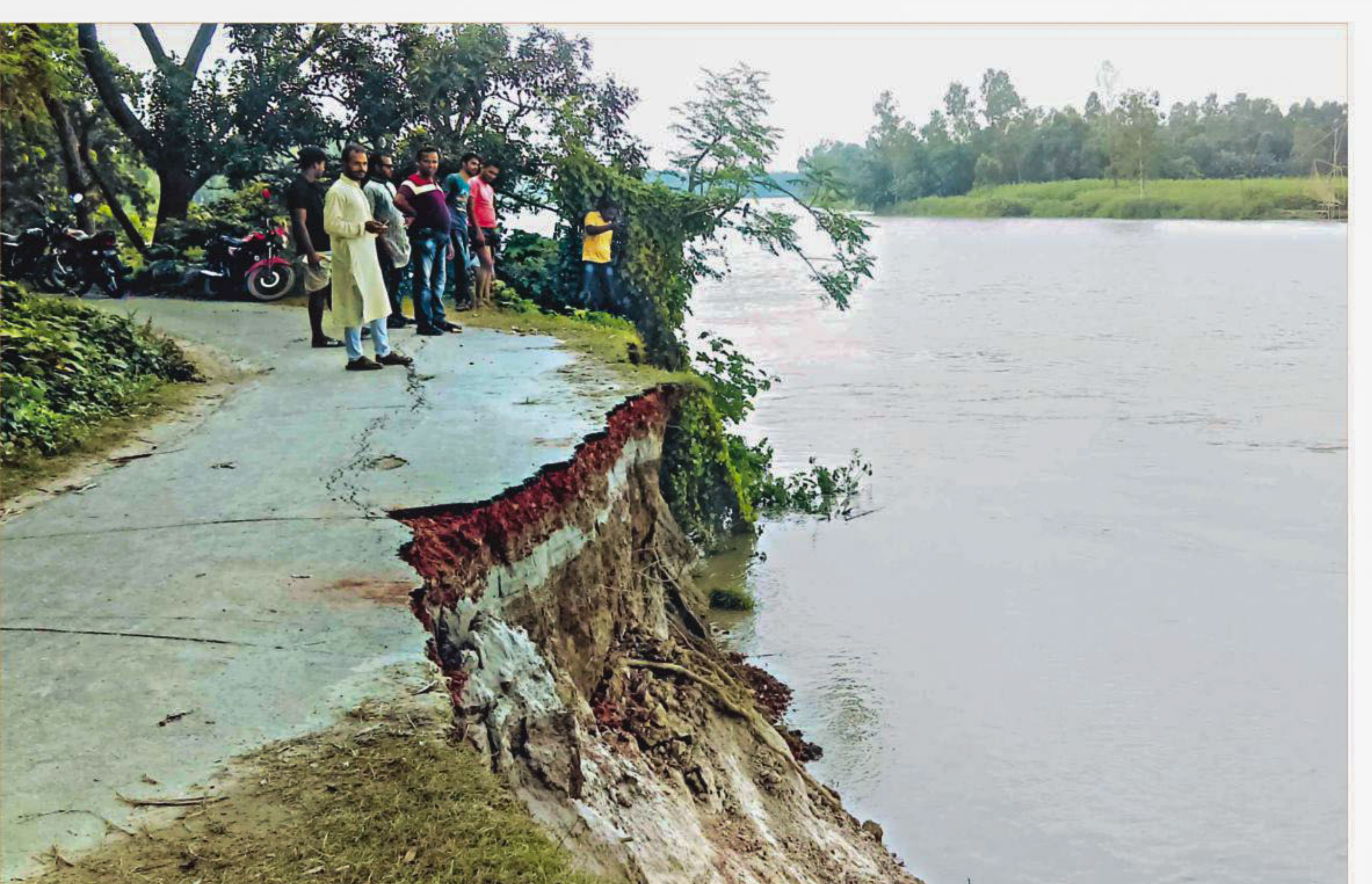
A portion of the damaged levee at Ranagachha village by the Jhinai river. PHOTO: MIRZA SHAKIL
