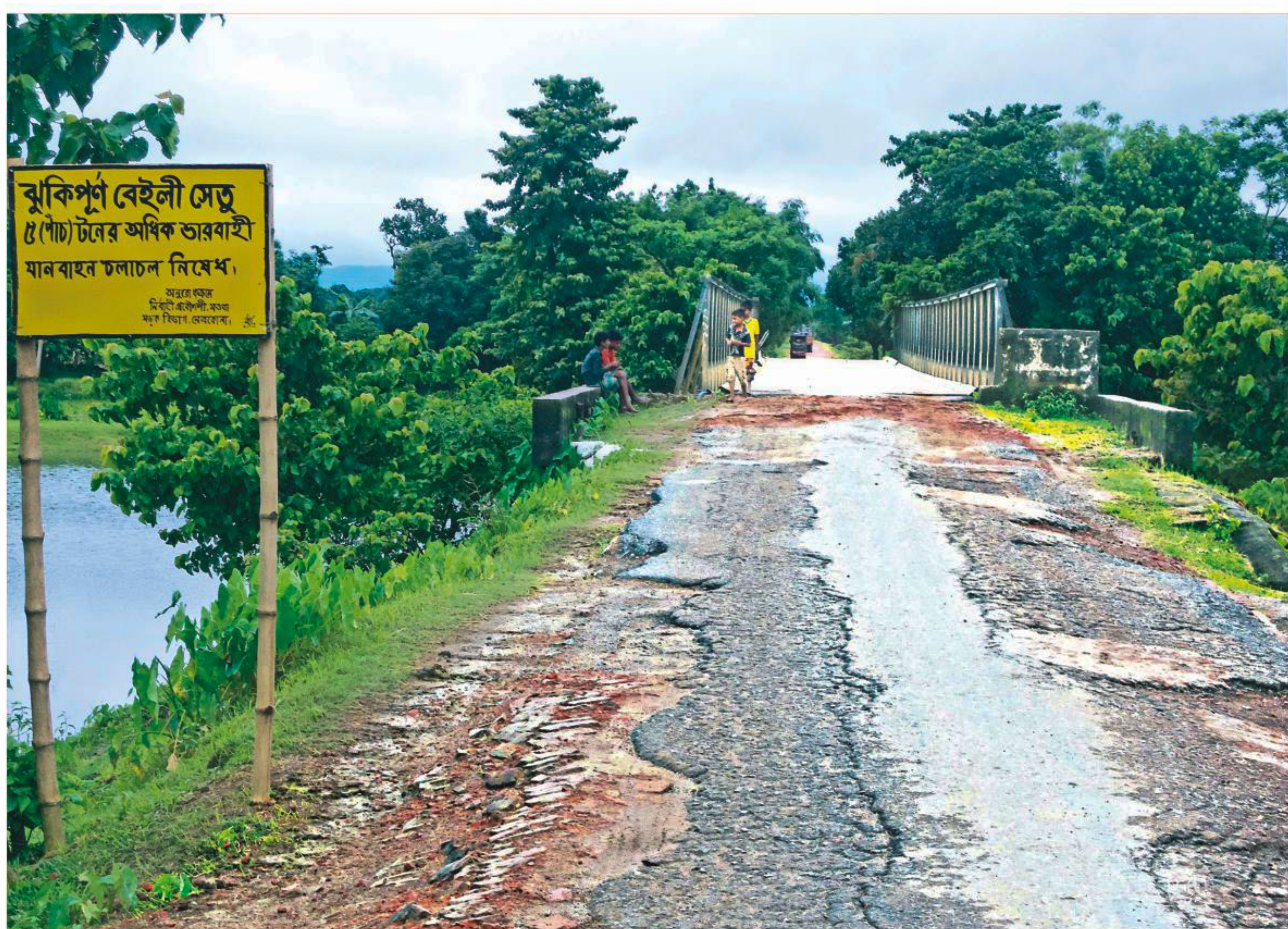
Kalmakanda-Thakurkona road in Netrakona remains in awful condition for years. The photo was taken from Babni area of Kalmakanda upazila a few days ago.
