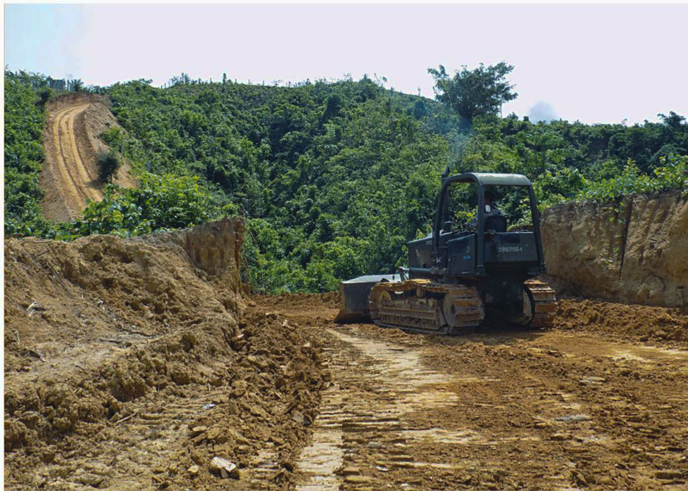
A hill is being razed with a bulldozer in Bandarban's Bir Bahadur Nagar area to build a road to a housing project, named after Bir Bahadur Ushwe Sing, state minister for Chittagong Hill Tracts affairs. The photo was taken early last month.
