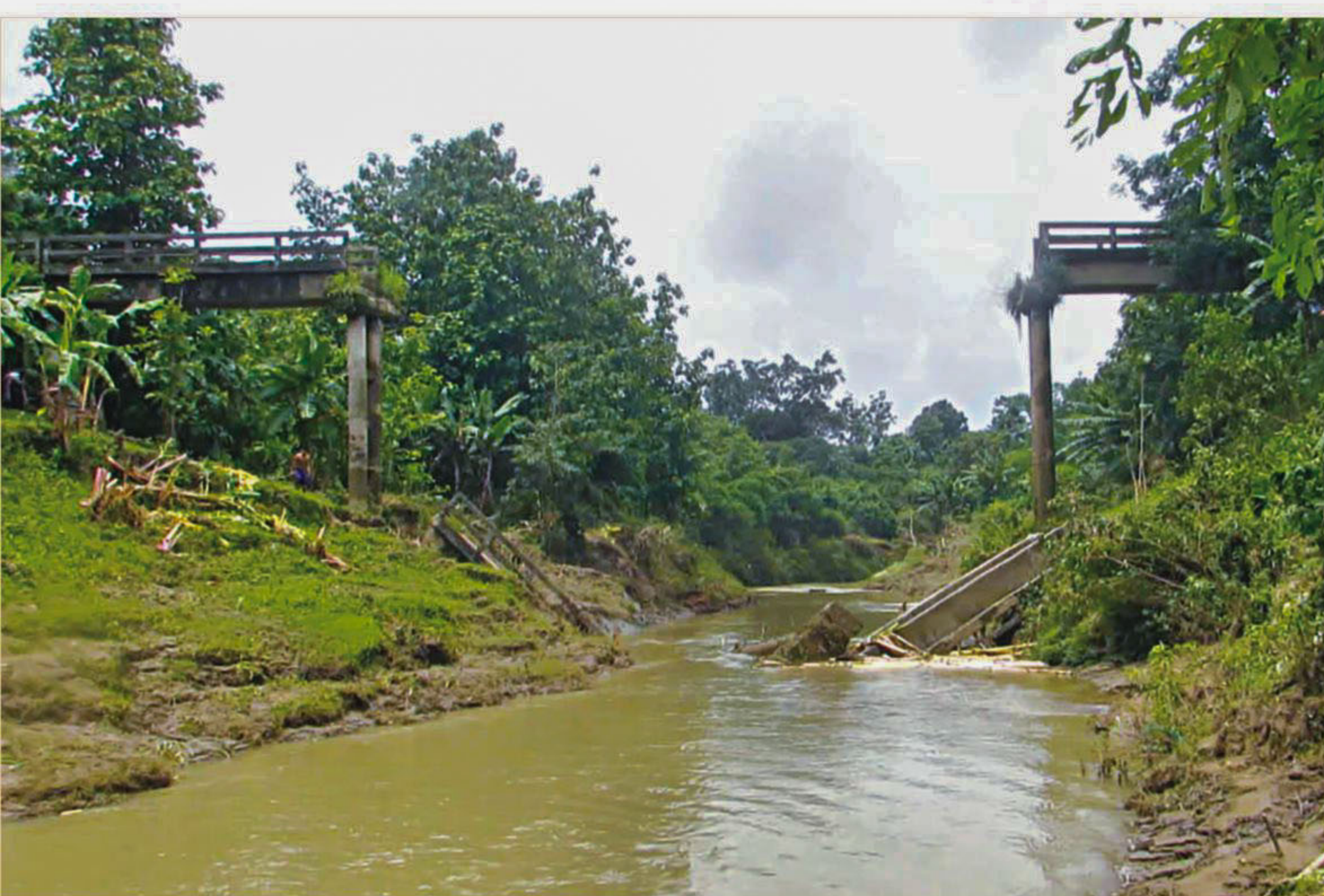
This bridge on a canal in Joutha Khamar area in Matiranga upazila of Khagrachhari collapsed on June 12, causing immense suffering to the people of the remote hill area.
