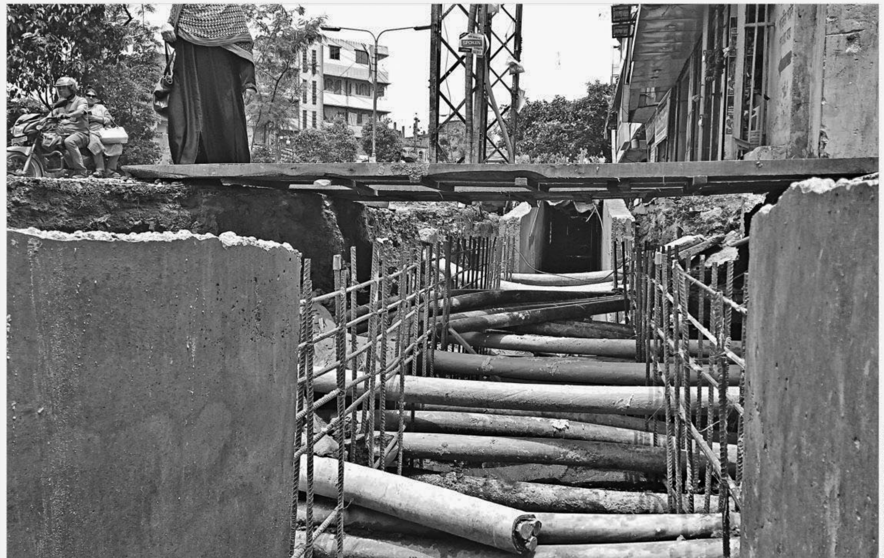
A deep drain is dug on the Mohammadpur end of the capital's Satmasjid Road -- right through high-voltage power lines of a sub-station of Dhaka Power Distribution Company (DPDC), exposing the wire lines as part of the construction. The photo was taken yesterday.
