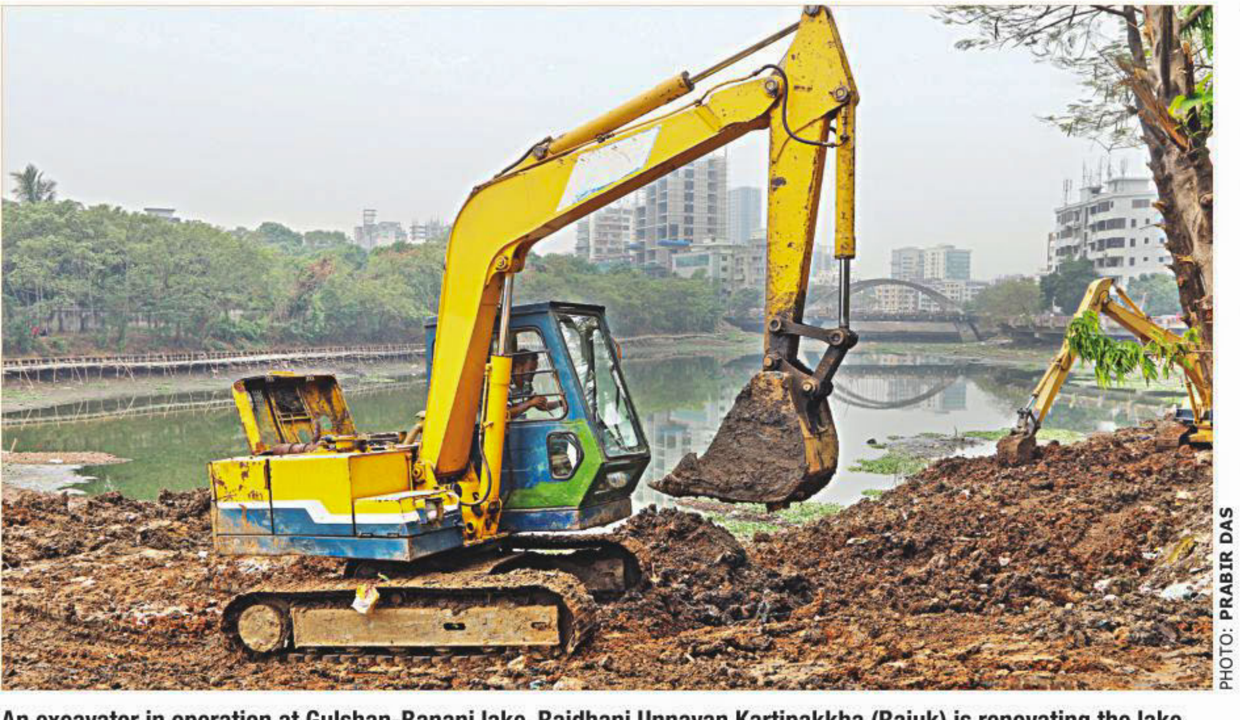
An excavator in operation at Gulshan-Banani lake. Rajdhani Unnayan Kartipakkha (Rajuk) is renovating the lake as part of its beautification project centring the lake. The photo was taken from Banani Bridge yesterday.
