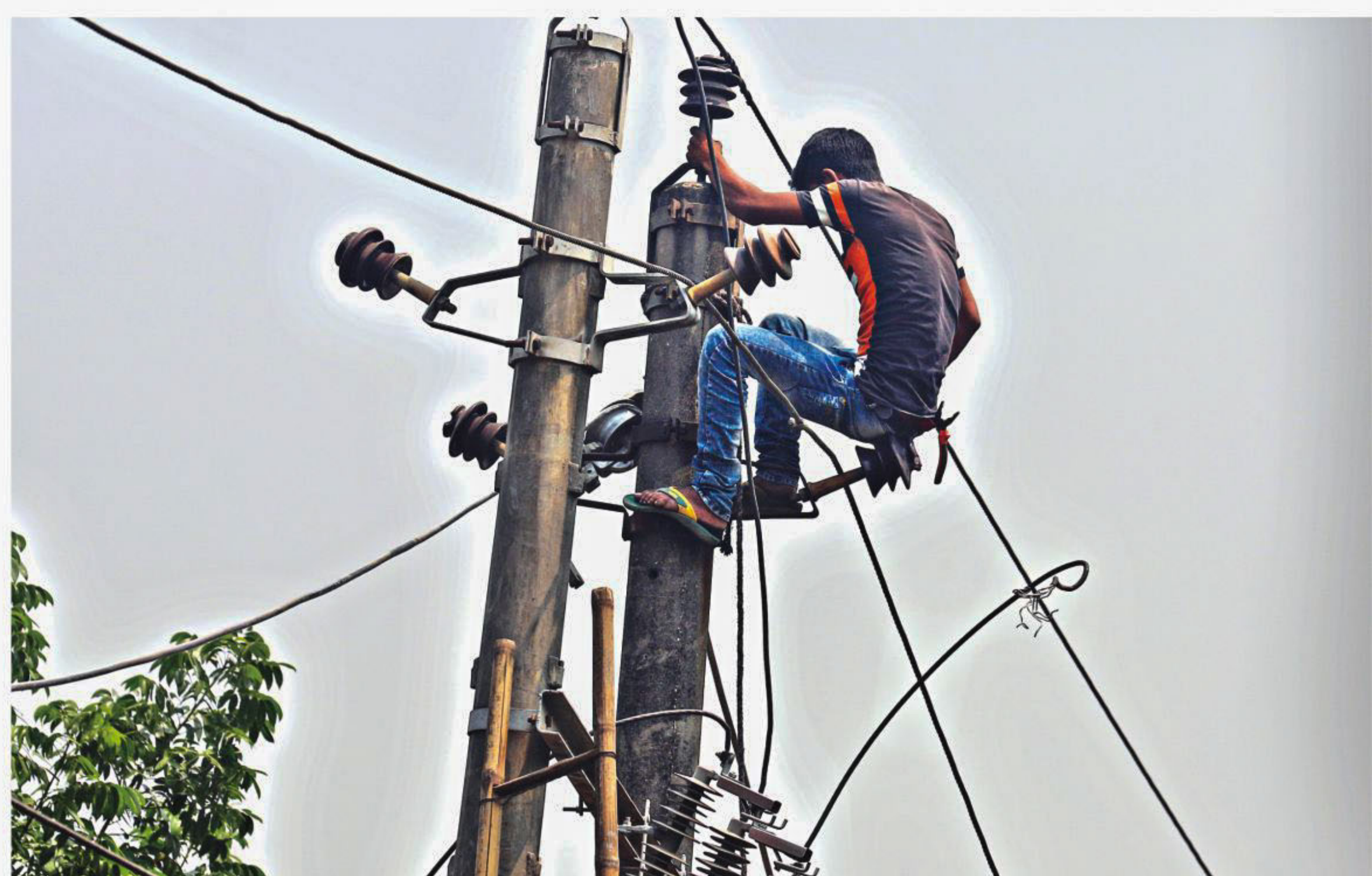
Showing blatant disregard for safety, an electrician is working on an electricity pole without any safety equipment. The photo was taken near Holy Cross Girls' High School in the city's Tejgaon area yesterday.
