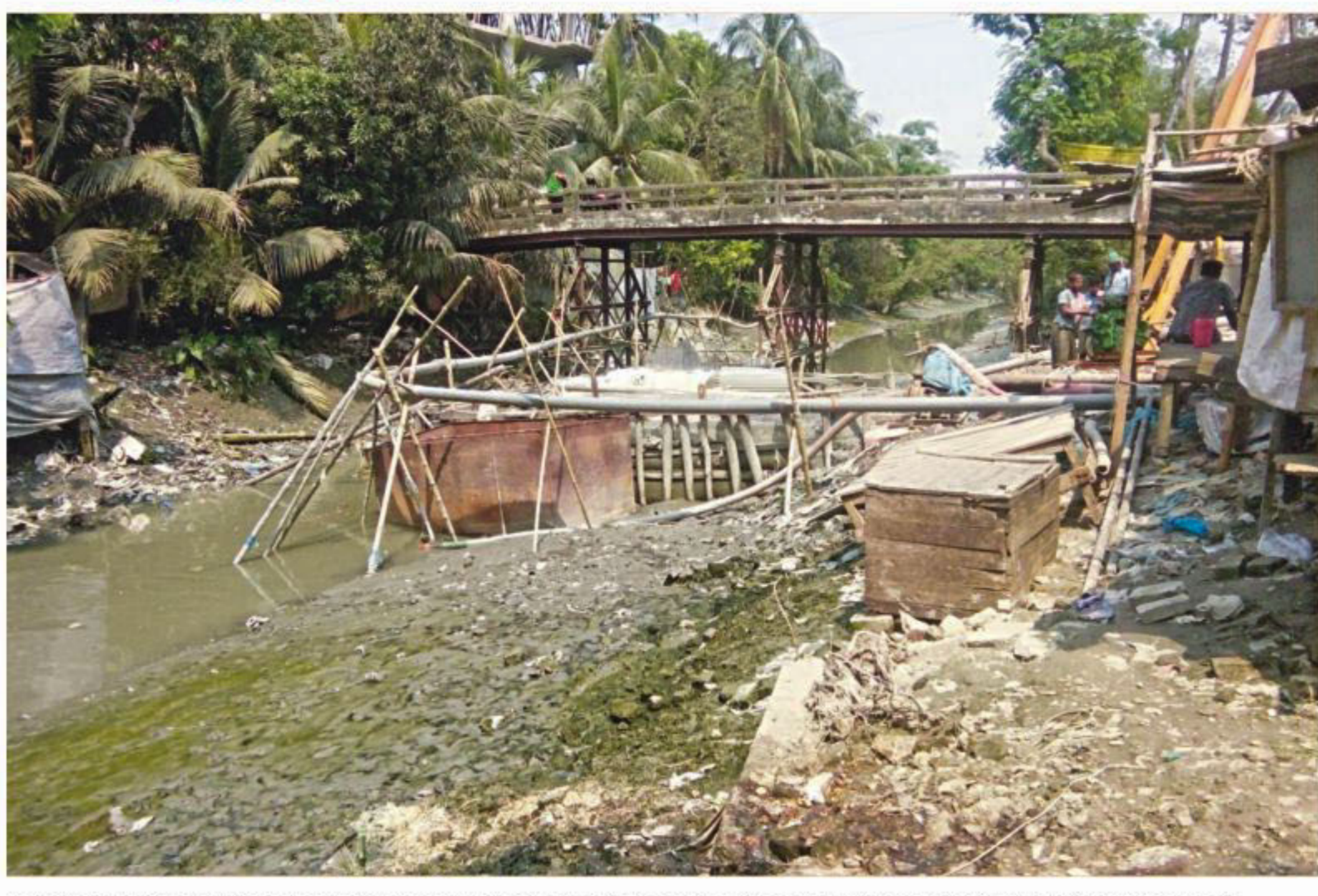
A ghatla (landing spot) under construction on Rajapur canal in the name of bazar development project in Rajapur upazila of Jhalakathi. The photo was taken from Rajapur Bazar recently. PHOTO: M JAHIRUL ISLAM JEWEL
