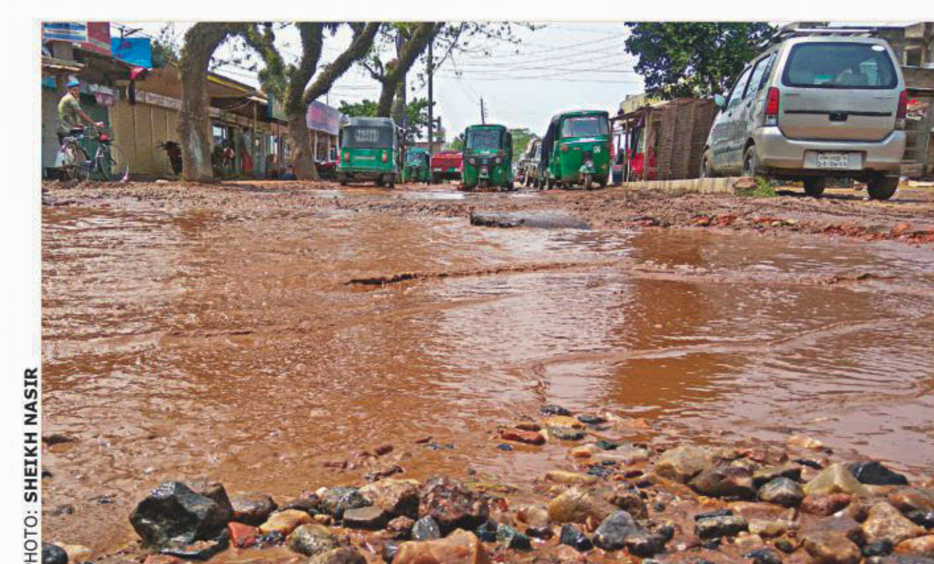
Commuters and pedestrians suffer on the battered and half-submerged Sylhet-Kanaighat-Burhanuddin road, which is a major artery joining Sylhet Sadar with Kanaighat and Golapganj upazilas. Due to lack of maintenance and disregard by the authorities, the road has developed many potholes making it extremely difficult for regular travel. The photo was taken yesterday in Muradnagar Bazar area.
