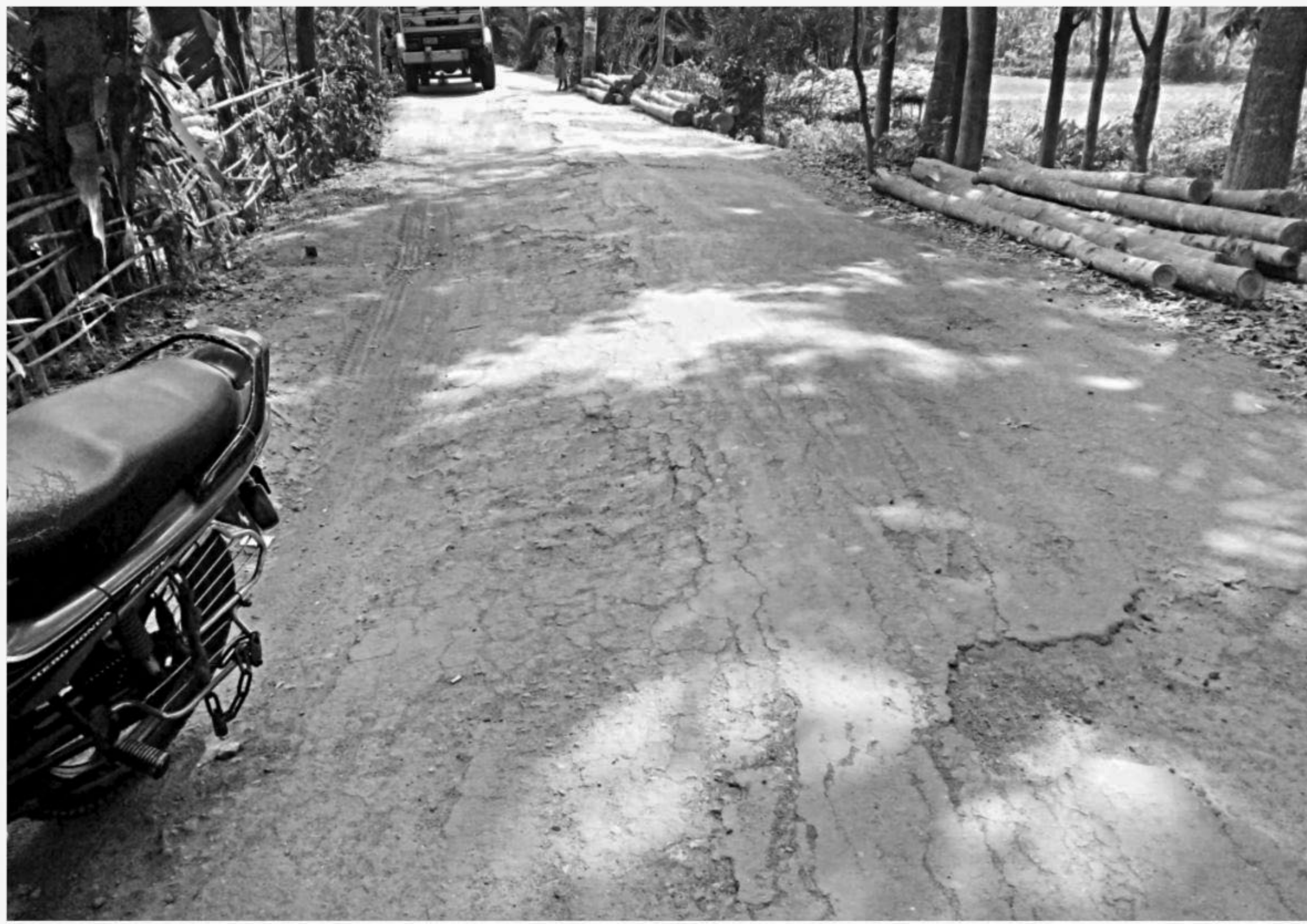
A portion of the damaged Amua-Kathalia-Rajapur-Jhalakathi road. The photo was taken at Angaria village in Rajapur upazila of Jhalakathi recently.
