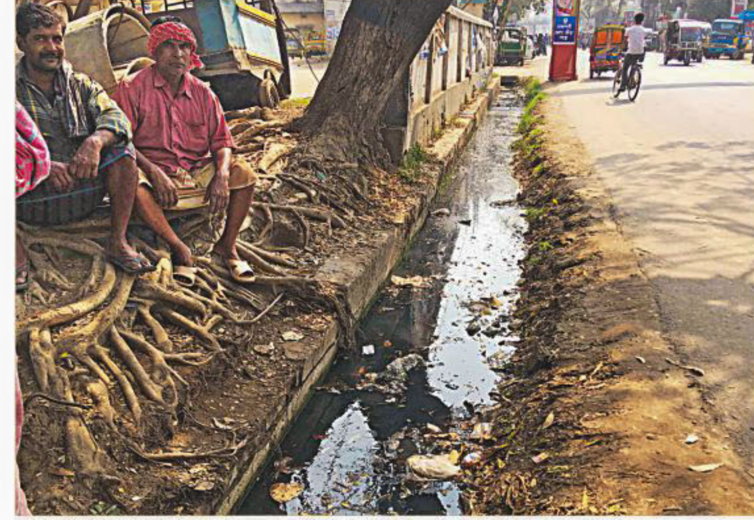
This is one of the many clogged up drains that has become a mosquito breeding ground in Rajshahi city. The photo was taken near Gourhanga intersection recently.
