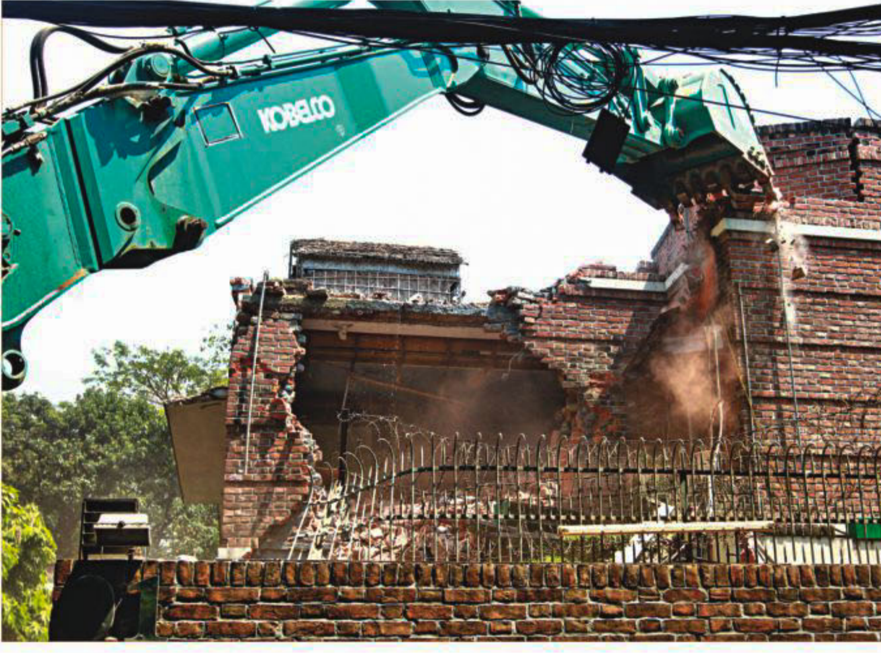
A hydraulic excavator is being used to tear down a section of AK Azad's house at Gulshan in the capital yesterday during a drive conducted by Rajdhani Unnayan Karttripakkha.
