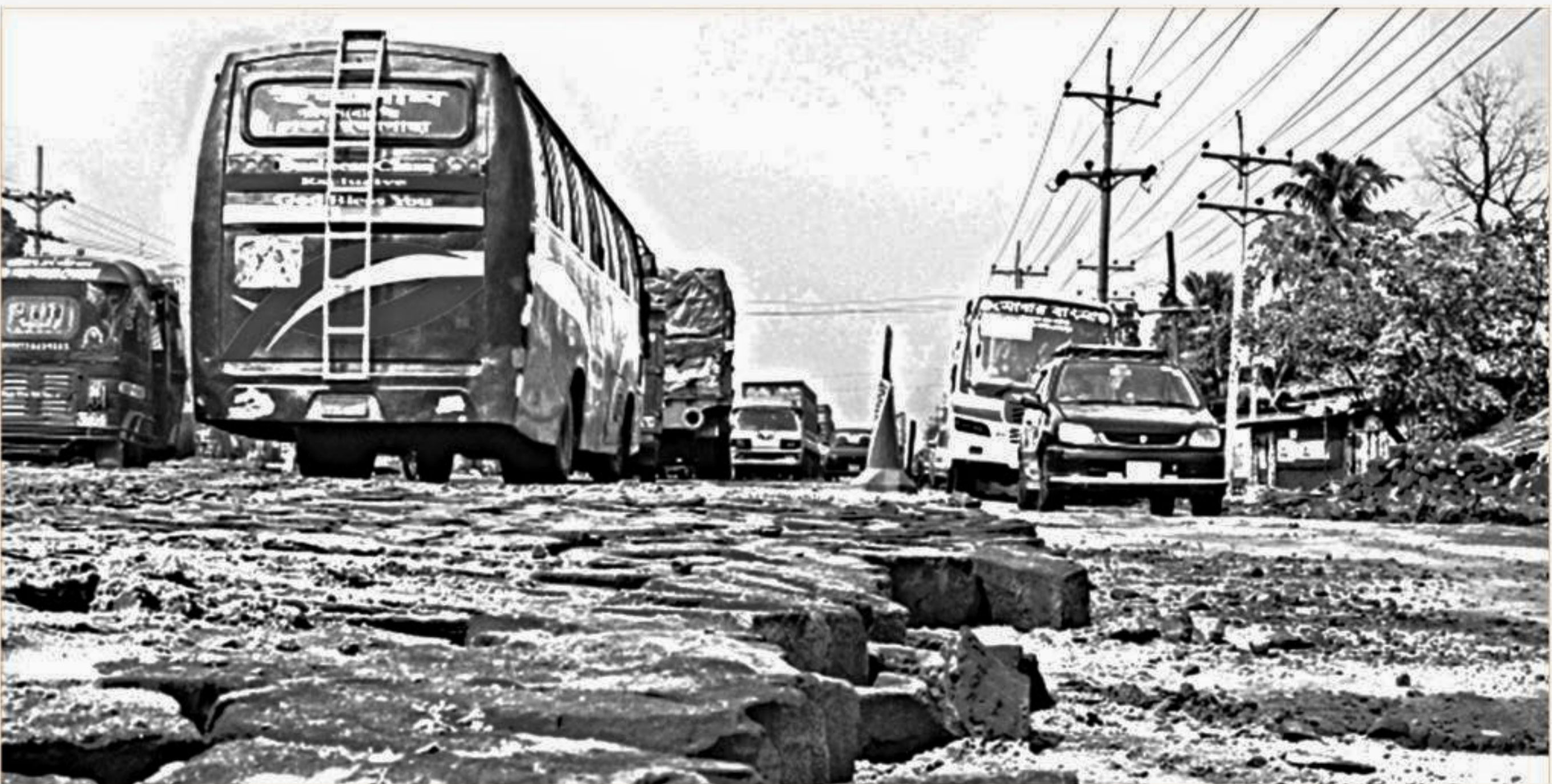
Only bricks have been laid on a portion of Dhaka-Mymensingh highway at Nog of Gazipur making it extremely difficult for vehicles to ply on them.
