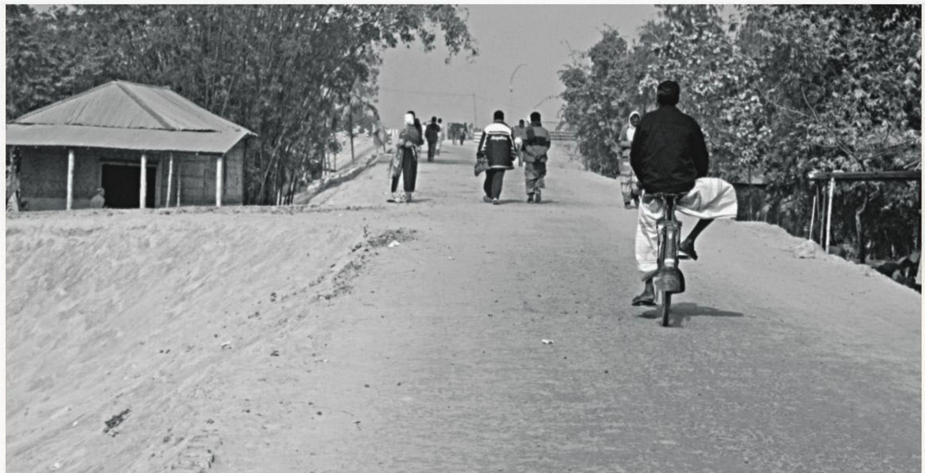
The 500-metre-long approach road of newly-built second Teesta Bridge on Kakina-Mahipur road in Kaliganj upazila of Lalmonirhat has been built with sand instead of earth. PHOTO: STAR
