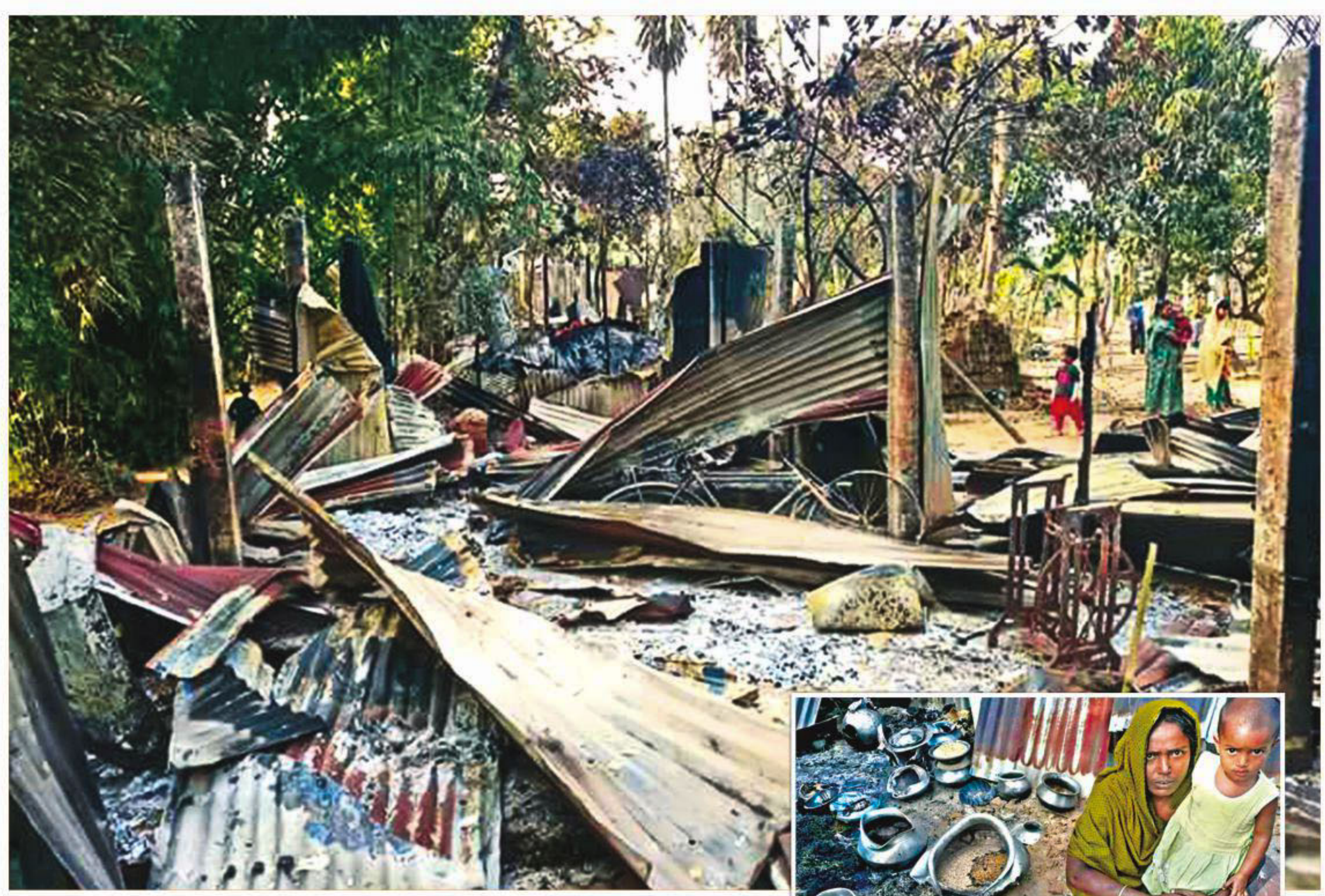
Arson-damaged houses in Ambari village of Sylhet's Jaintiapur upazila. Around 45 houses were torched by criminals in three villages of the upazila early on Monday after a clash had broken out between two groups of locals over organising a waz mehfil in Ambari, some 30 kilometres off Sylhet city. PHOTO: COLLECTED
