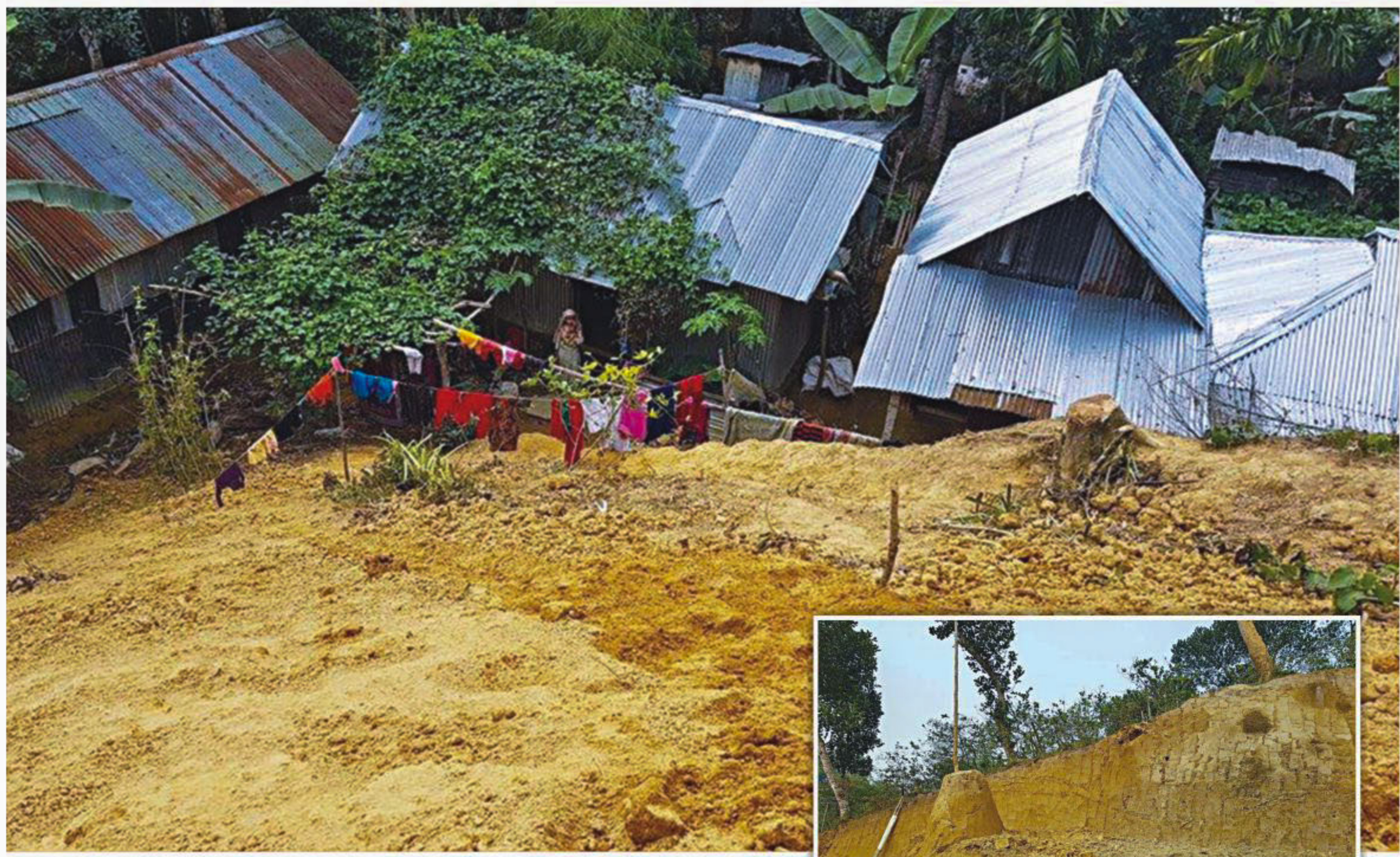
Due to illegal hill cutting, many families living in the slopes of the hills at Bishamoni village in Moulvibazar's Sreemangal upazila are exposed to mudslides during the rainy season. Inset, cutting of hills goes unabated, violating environmental laws.
