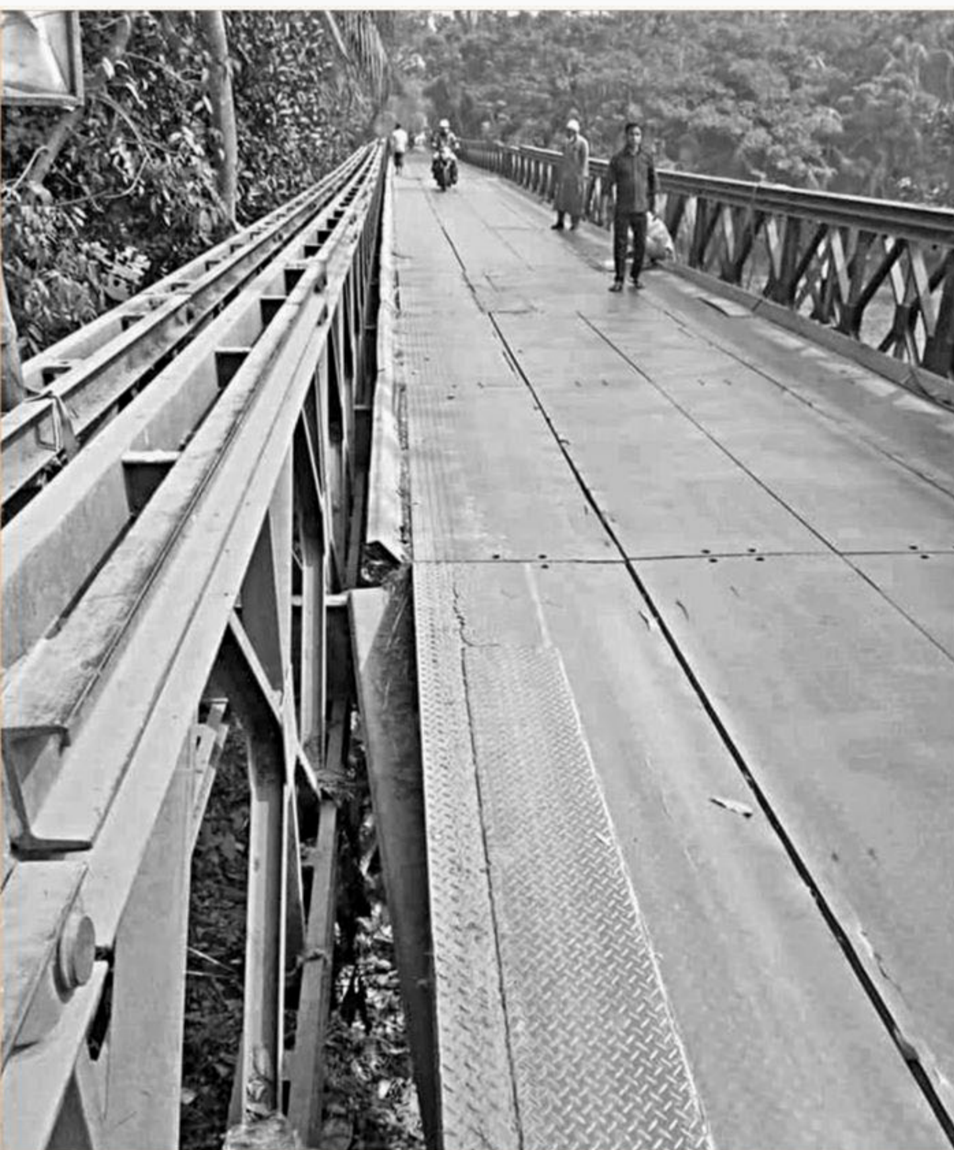
This Bailey bridge on Guthia canal in Barisal's Babuganj upazila has become awfully risky for its users as some of its steel decks are badly damaged and displaced.
