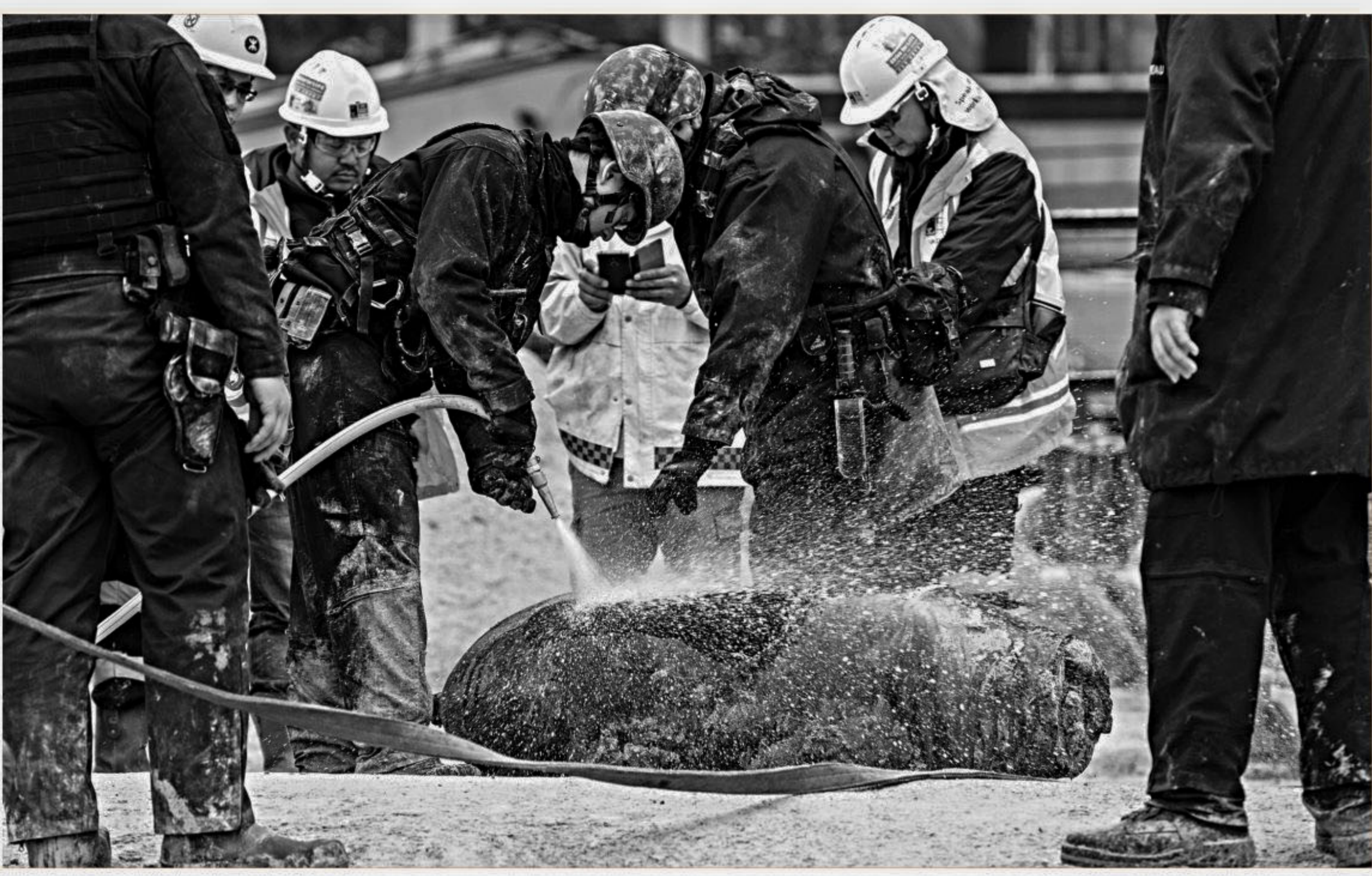
Police from the explosive ordinance disposal unit hose down a defused US-made bomb dropped during World War II a day after it was discovered on a harbour front construction site in the Wan Chai district of Hong Kong yesterday.
