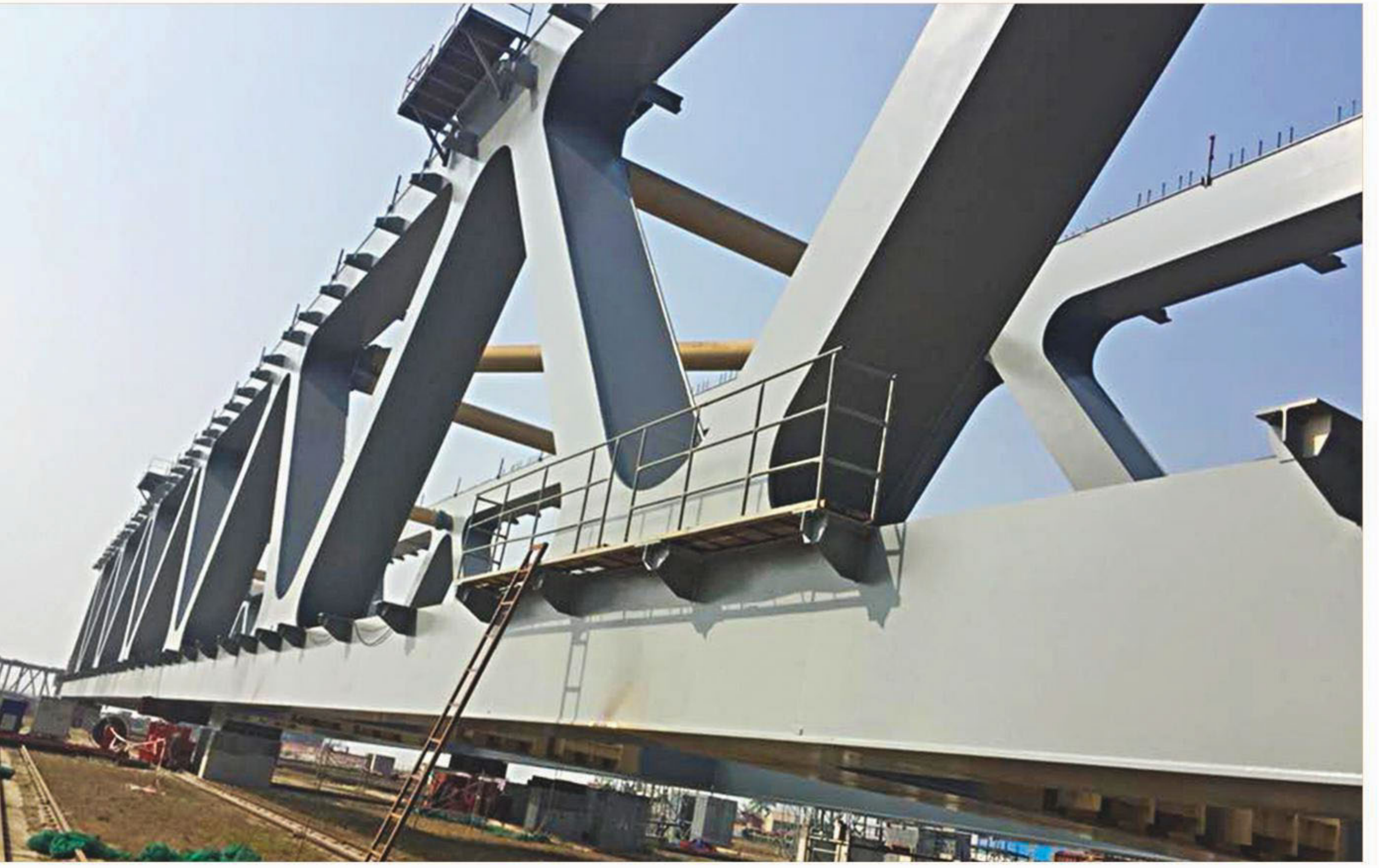
The second span (superstructure) of the Padma Bridge at the bridge construction site at Kumarbhog in Munshiganj recently. It will be on its way to the Jajira point in Shariatpur today and installed by this month. The first span was put up in September last year. With a total of 41 such spans, the two-level bridge will carry a four-lane highway on the upper level and a single track railway on the lower level.
