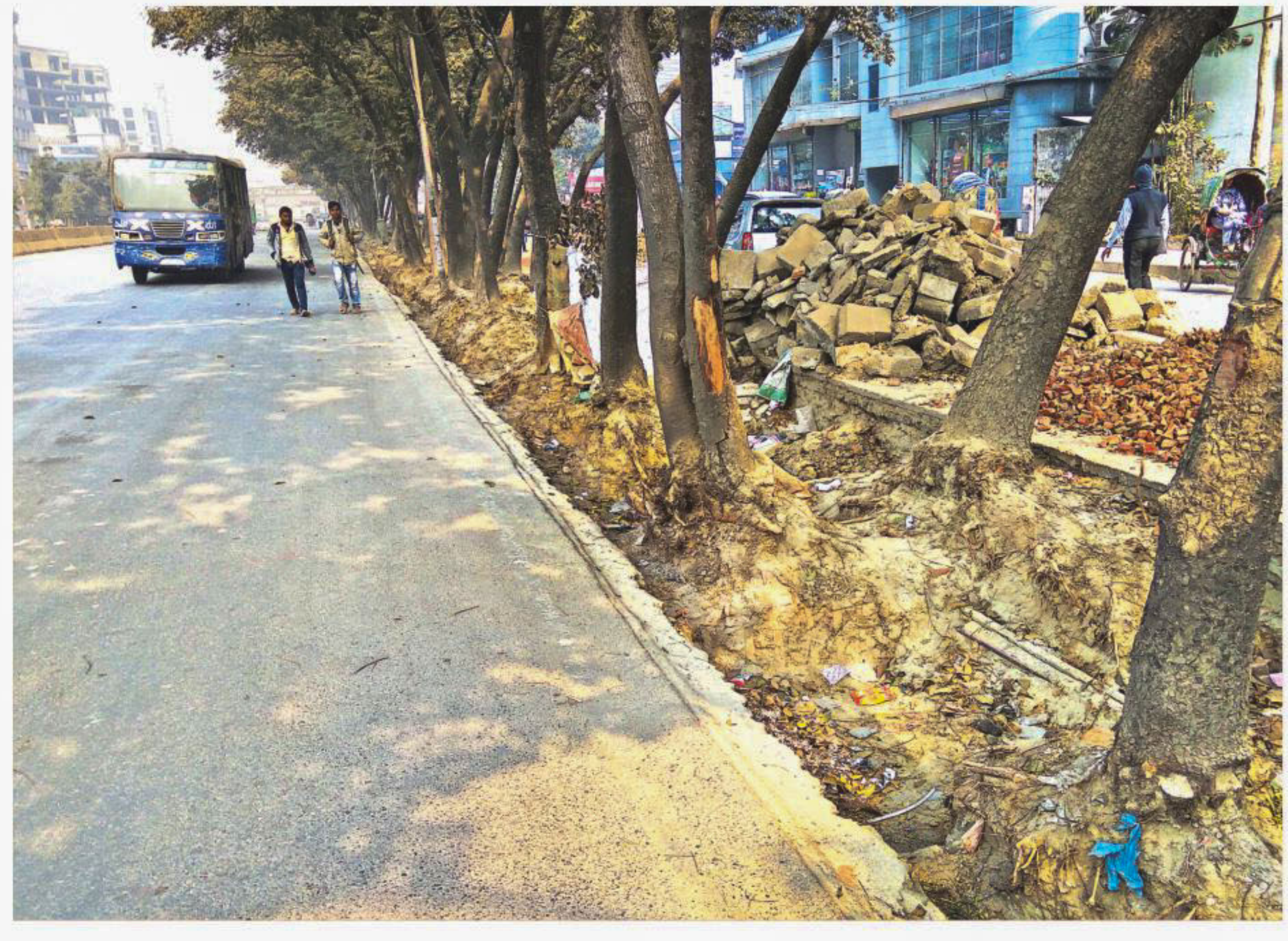
As the footpath is dug up for a "development project", two pedestrians walk on the busy road while a speeding bus passes by. In such scenario, fatal accident can happen in a fraction of a second. Moreover, there is no sign warning the approaching vehicles of the trench right beside the road. In addition, roots of the trees beside the road get exposed as the soil has been removed. As a result, some of the trees died, as said by locals. The photo was taken at Uttara Sector 4 in the capital yesterday.
