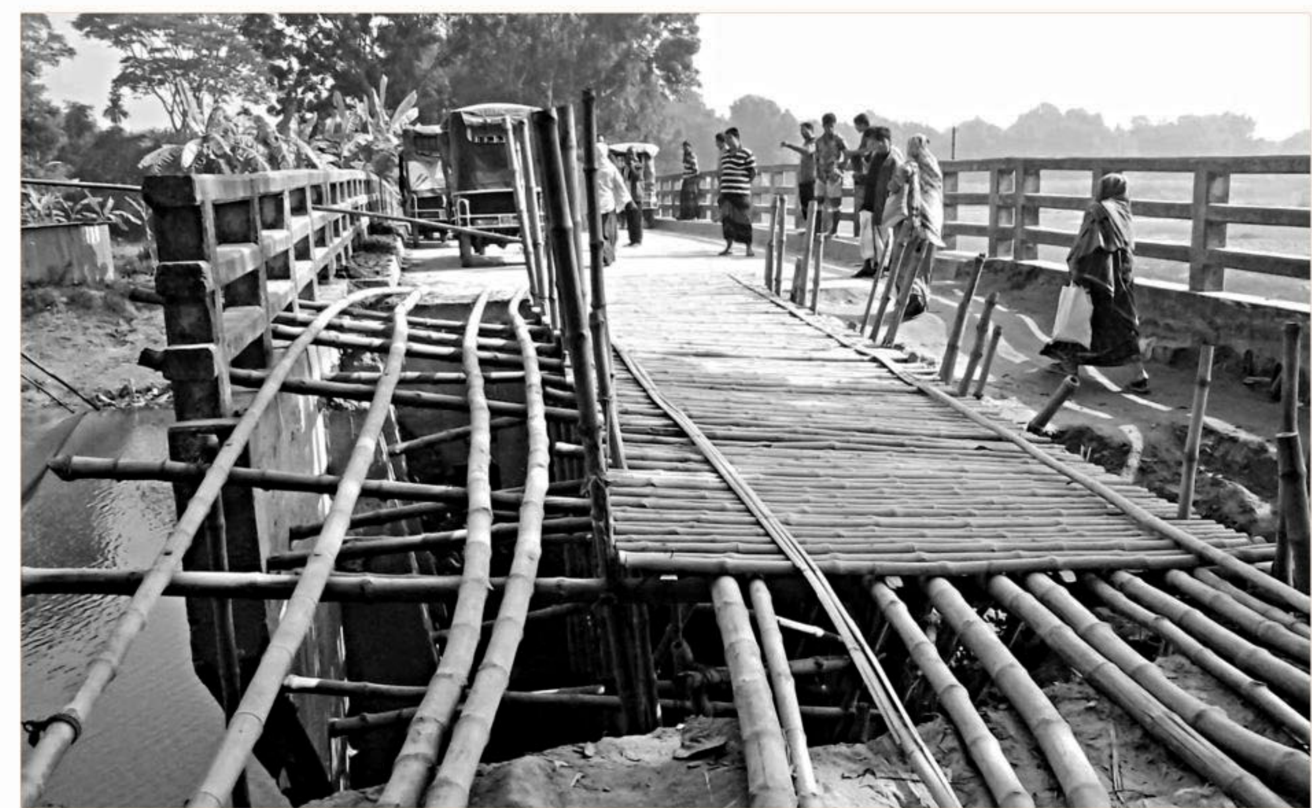
People cross the gap caused by collapse of the approach road to the bridge in Gorasin area under Delduar upazila of Tangail, using a bamboo platform.
