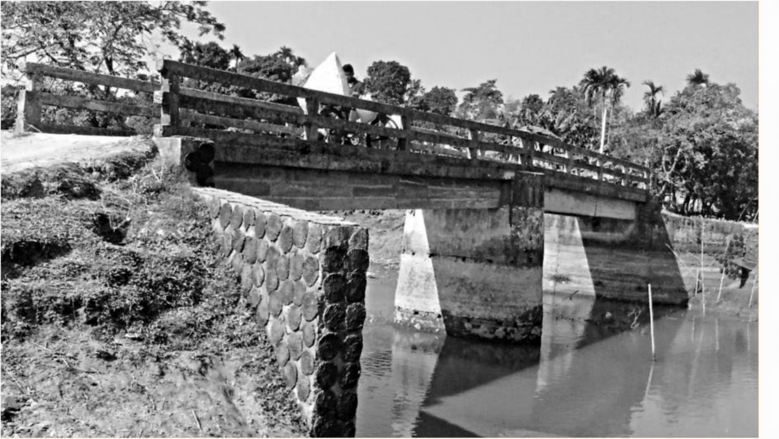
People of Dharakandi and Khalodbari villages in Maoha union of Gouripur upazila of Mymensingh built this bridge over the Suria river in six years through their own effort and money.
