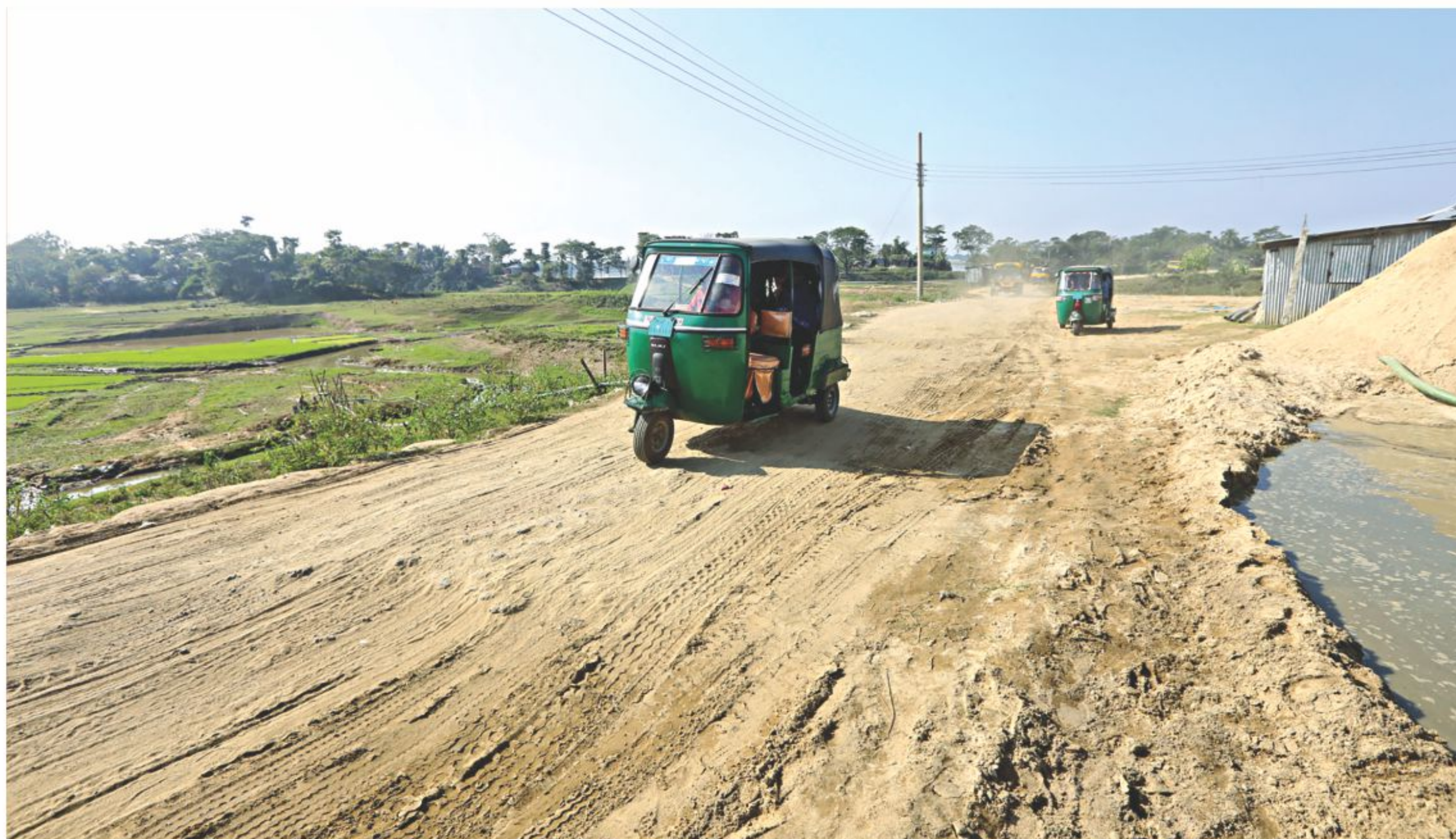
At first sight this might appear to be an under construction road. But in reality, this is a fully constructed road connecting Osmani International Airport, Badaghat and Kumargaon in Sylhet. Around Tk 27.5 crore was spent to complete the six-kilometre-long road seven years ago under a priority project of the local lawmaker. But before it could be inaugurated officially, asphalt layers from most parts of the road have dissipated. The photo was taken from Baish Tila area yesterday.
