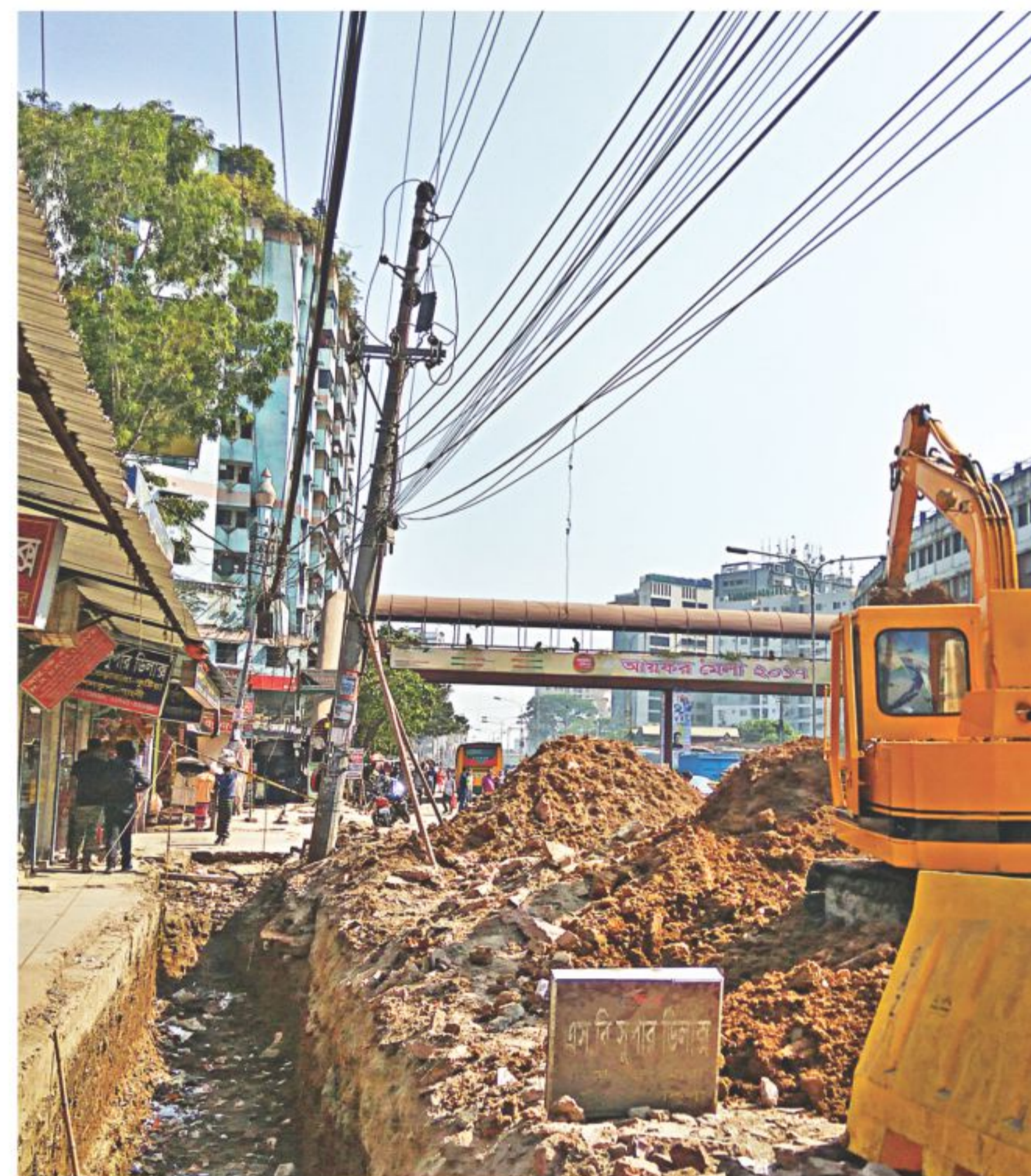
A tunnel dug along the Mirpur road so carelessly that it loosened earth at the base of an electric pillar, which supports a bundle of high-tension cables. Although the city corporation workers placed two bamboos to shore up the metal pillar, they may collapse under its load and cause casualties. The photo was taken in Kalyanpur on Wednesday.
