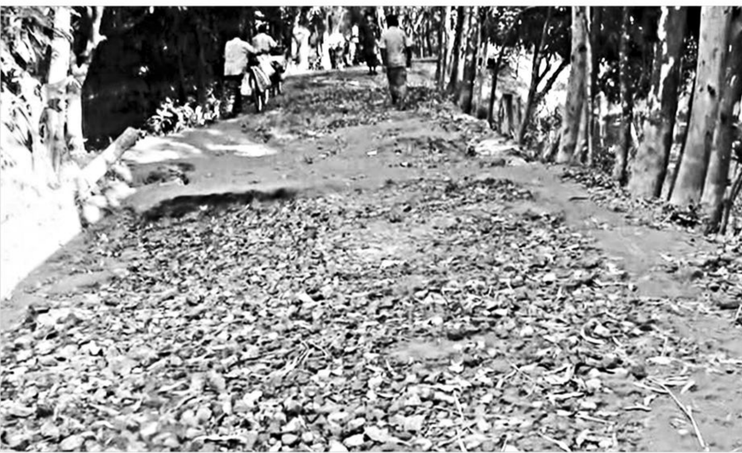
The surface of the paved road at Katir Haat in Fulchhari upazila of Gaibandha has been completely washed away by flood, hampering communication between many villages and the upazila headquarters.
