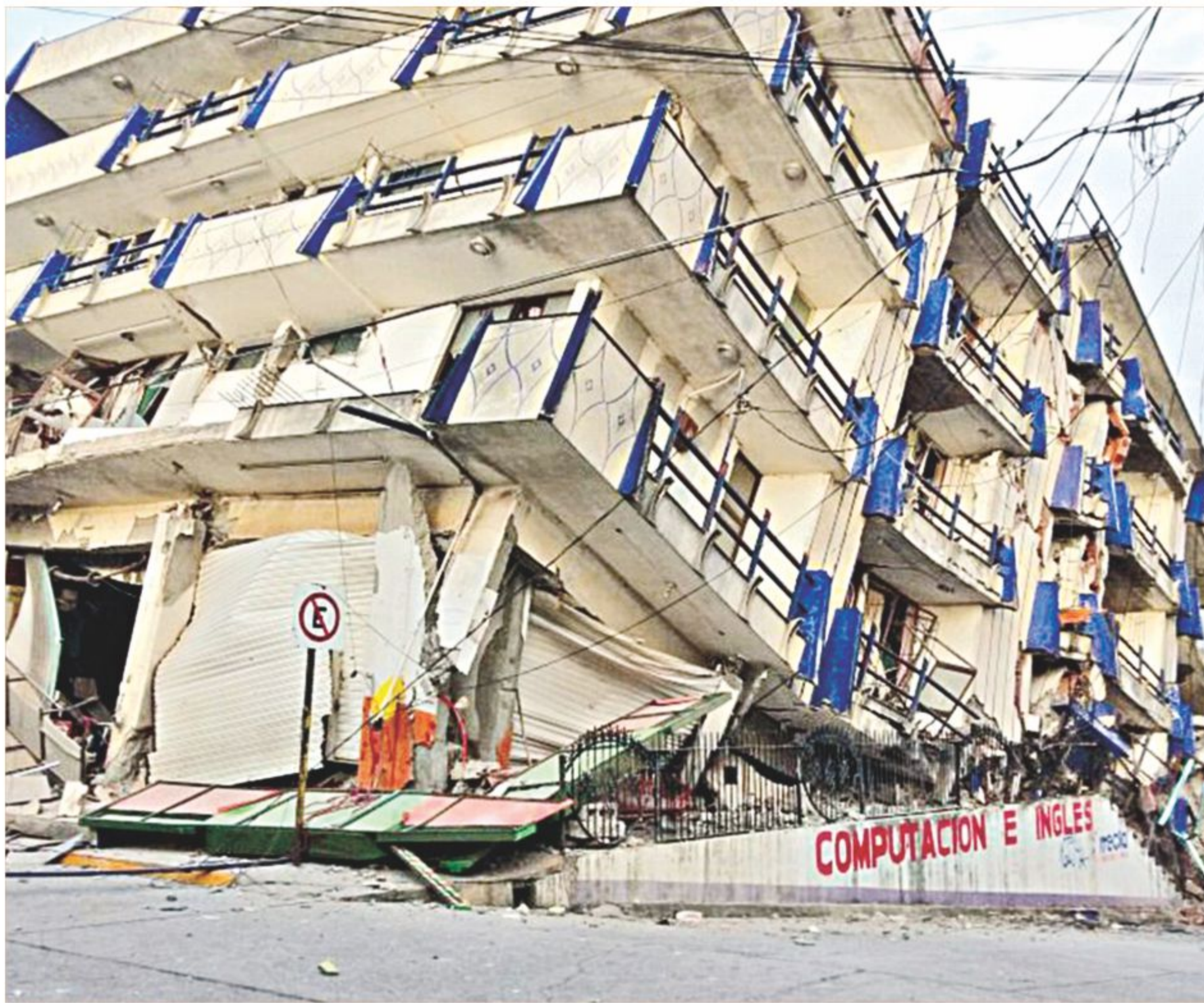
(Clockwise from left) A collapsed building in Juchitan in Oaxaca is pictured after an 8.1 magnitude earthquake hit Mexico late on Thursday; people gather on a street in downtown Mexico City during the earthquake.
