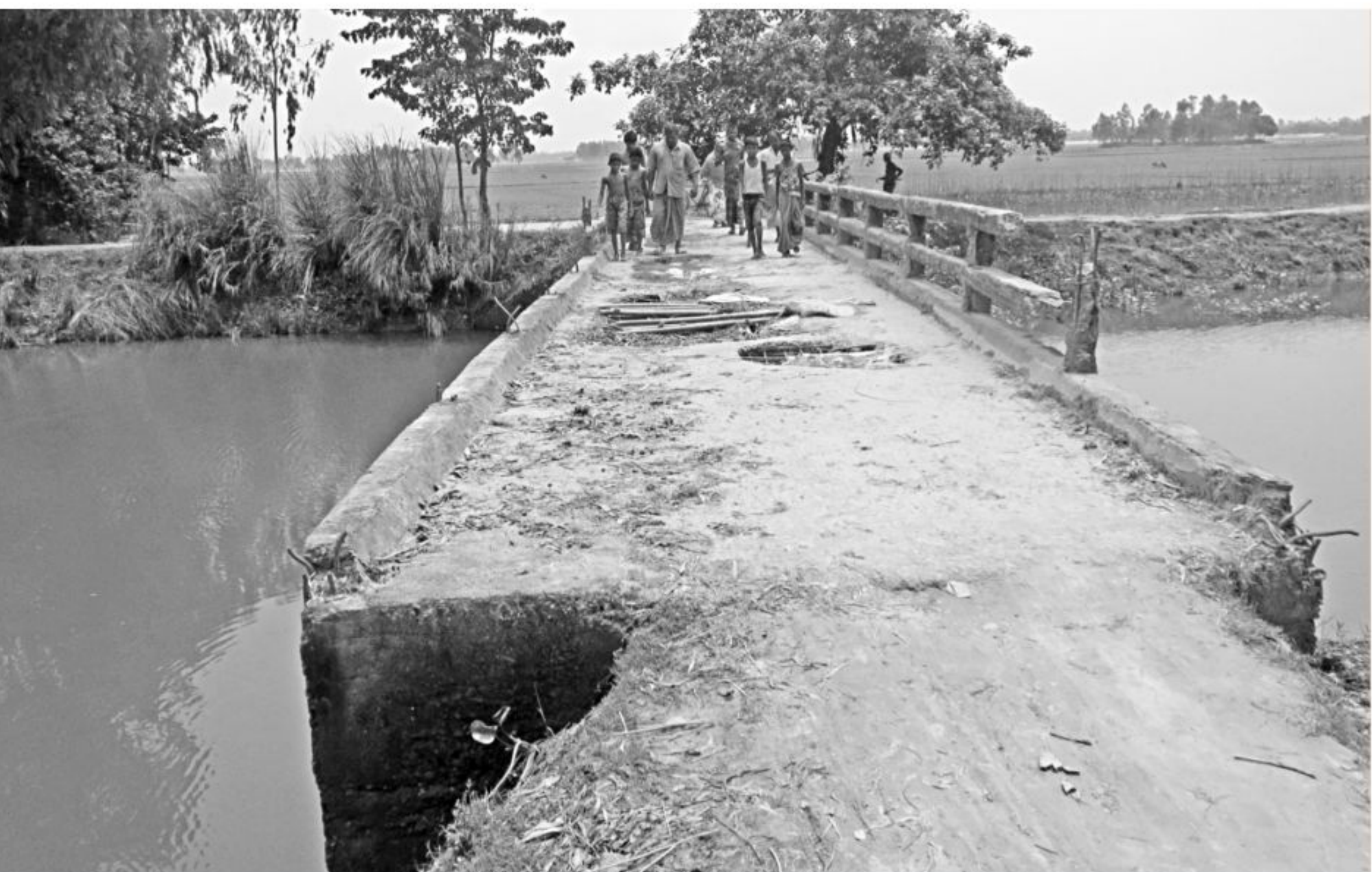
This bridge over Dikdari canal at Jhakuapara village in Kurigram's Nageshwari upazila has remained broken for five years, hampering communication between five unions and the upazila and district headquarters.
