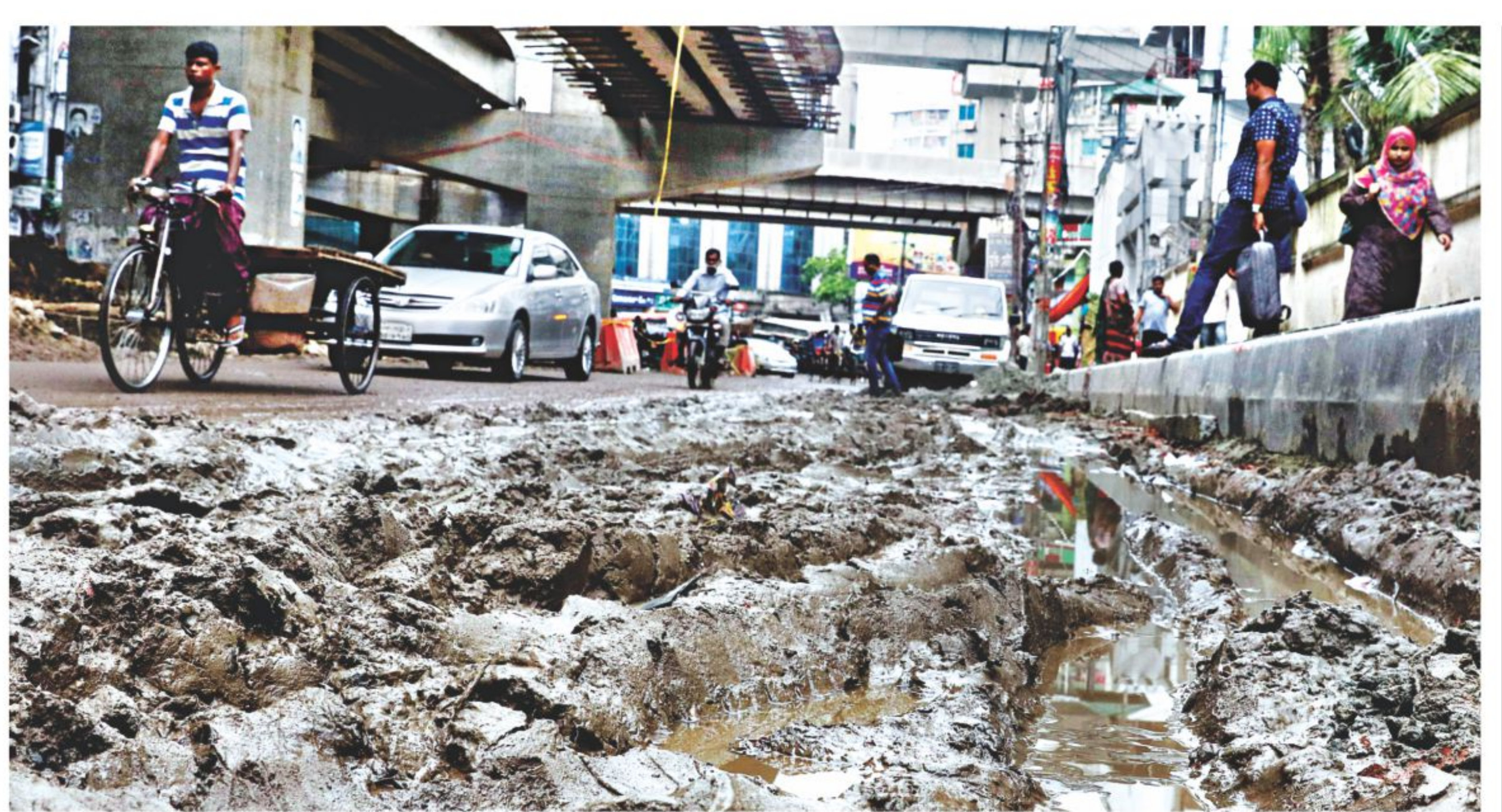
The damaged portion of this road hinders vehicular movement in the capital's Malibagh area. The road has been left unrepaired for a long time due to the work of Moghbazar-Mouchak flyover. The photo was taken recently.
