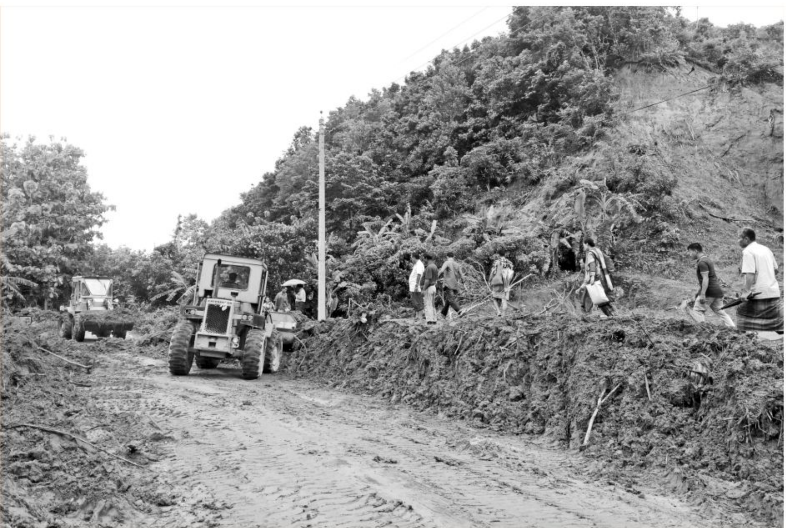
A landslide on June 13 severely damaged the Rangamati-Khagrachhari road, stopping traffic movement on the route. The photo was taken yesterday from Khamar Para area of Rangamati's Sapchhari union.
