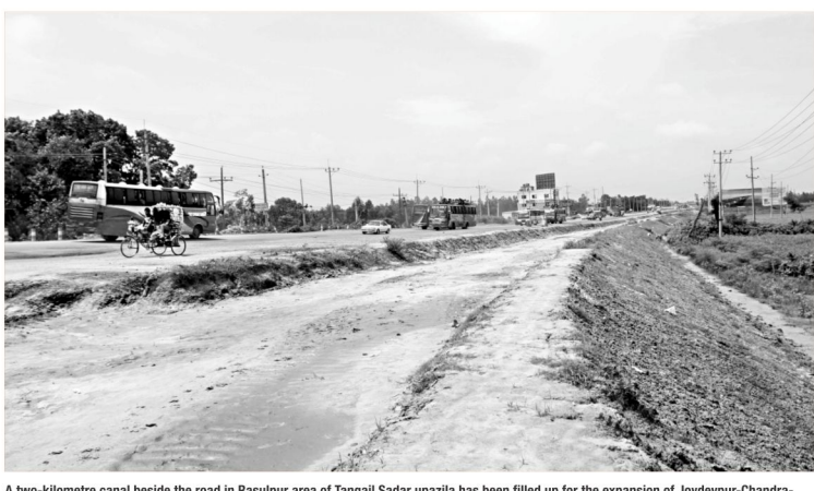
A two-kilometre canal beside the road in Rasulpur area of Tangail Sadar upazila has been filled up for the expansion of Joydevpur-Chandra-Tangail-Elenga highway into a four-lane road.
