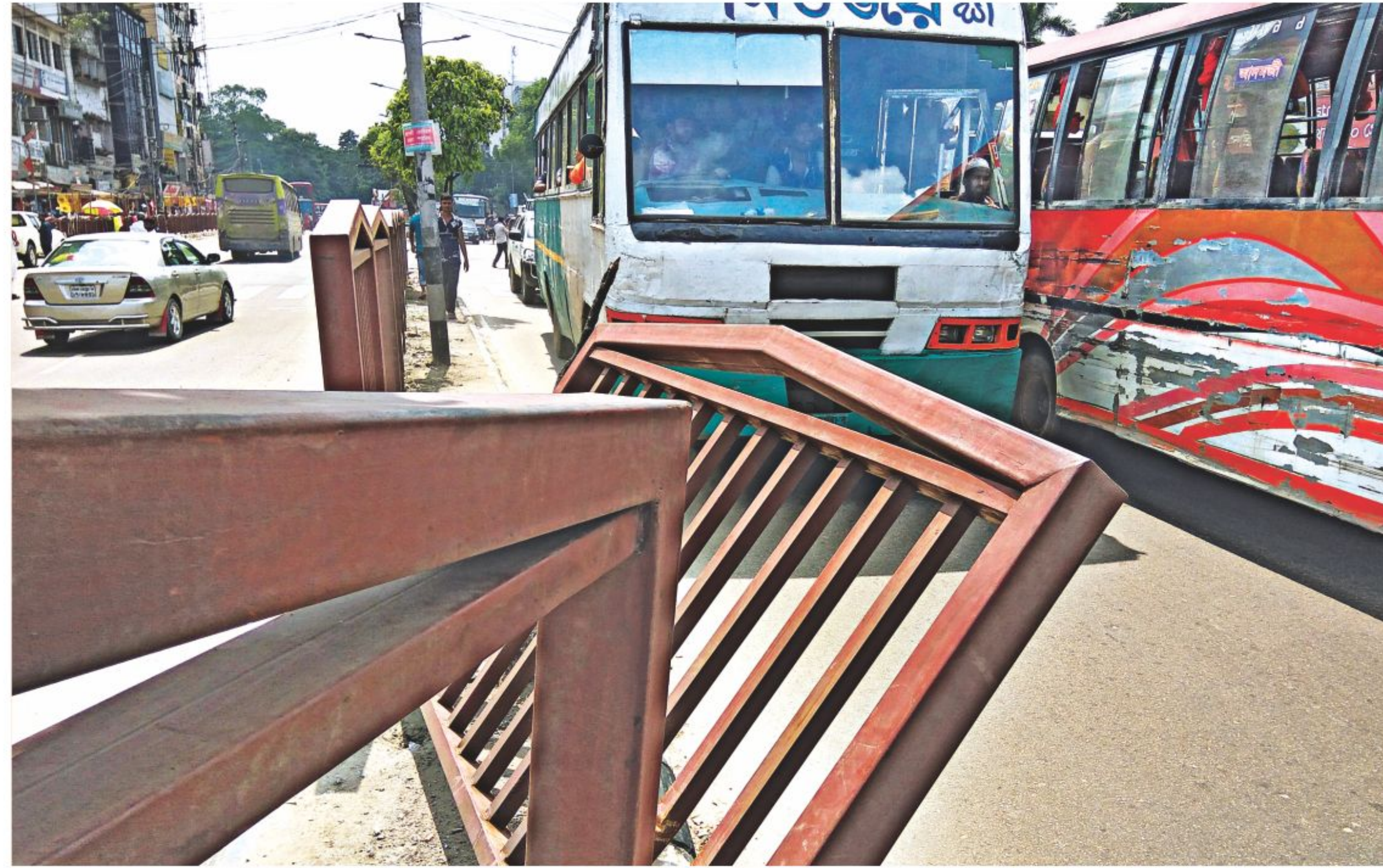
A metal road divider precariously leans toward a portion of Bangabandhu Avenue near GPO intersection in the capital. Locals said at least two such dividers have been in this state since a speeding vehicle hit those several nights back. The authorities apparently are yet to take notice.
