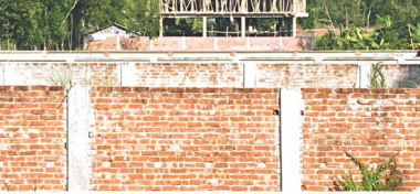
A structure being built without construction permits in Utaran Grehayan Samabay Samity in Cox's Bazar. The photo was taken recently. PHOTO: STAR
