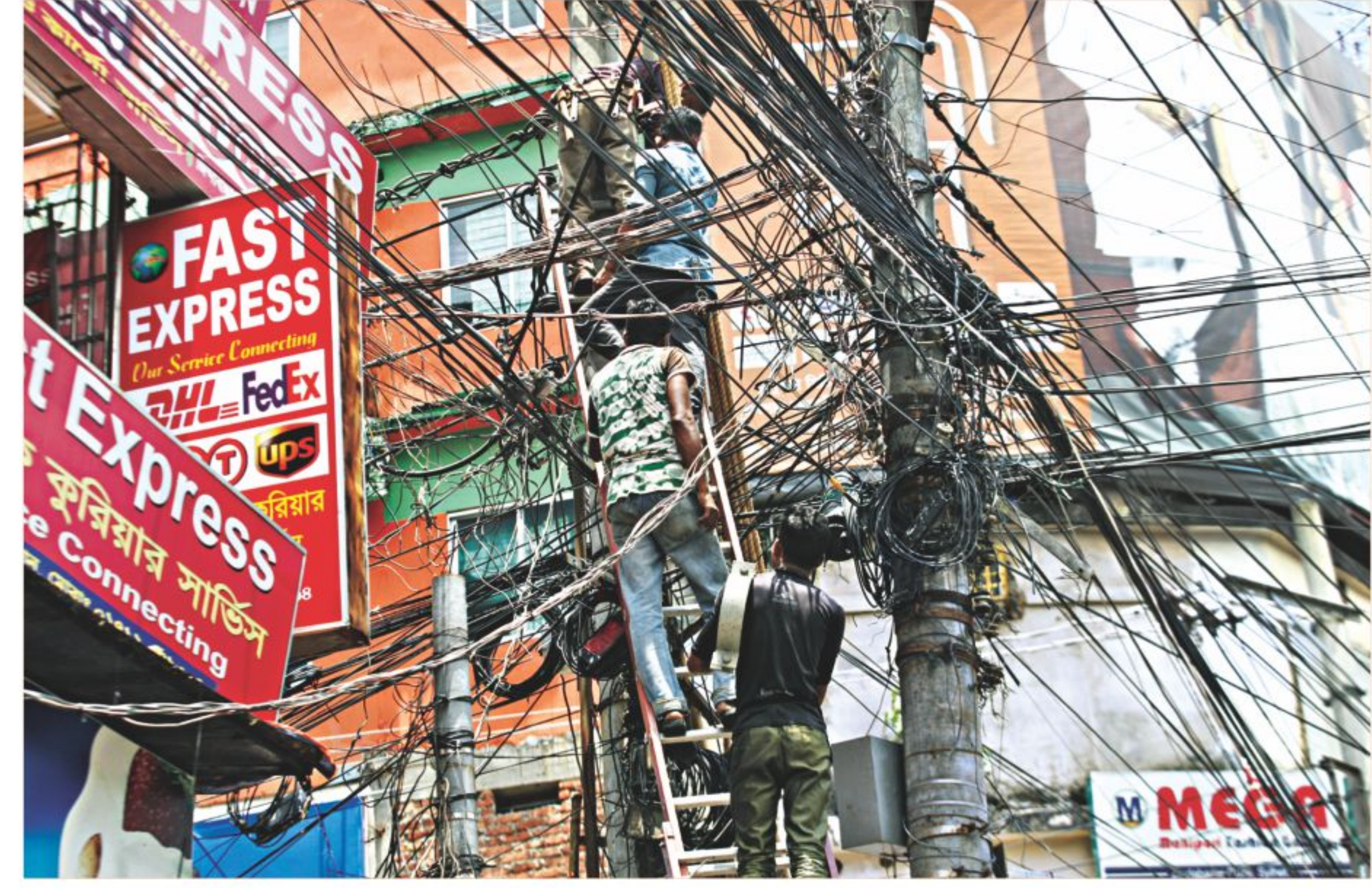
Four people working with different types of cables including of electricity in Zindabazar area in Sylhet city last week. Though the job is hazardous, sometimes fatal, both the workers and their employers seem to be equally indifferent to safety.
