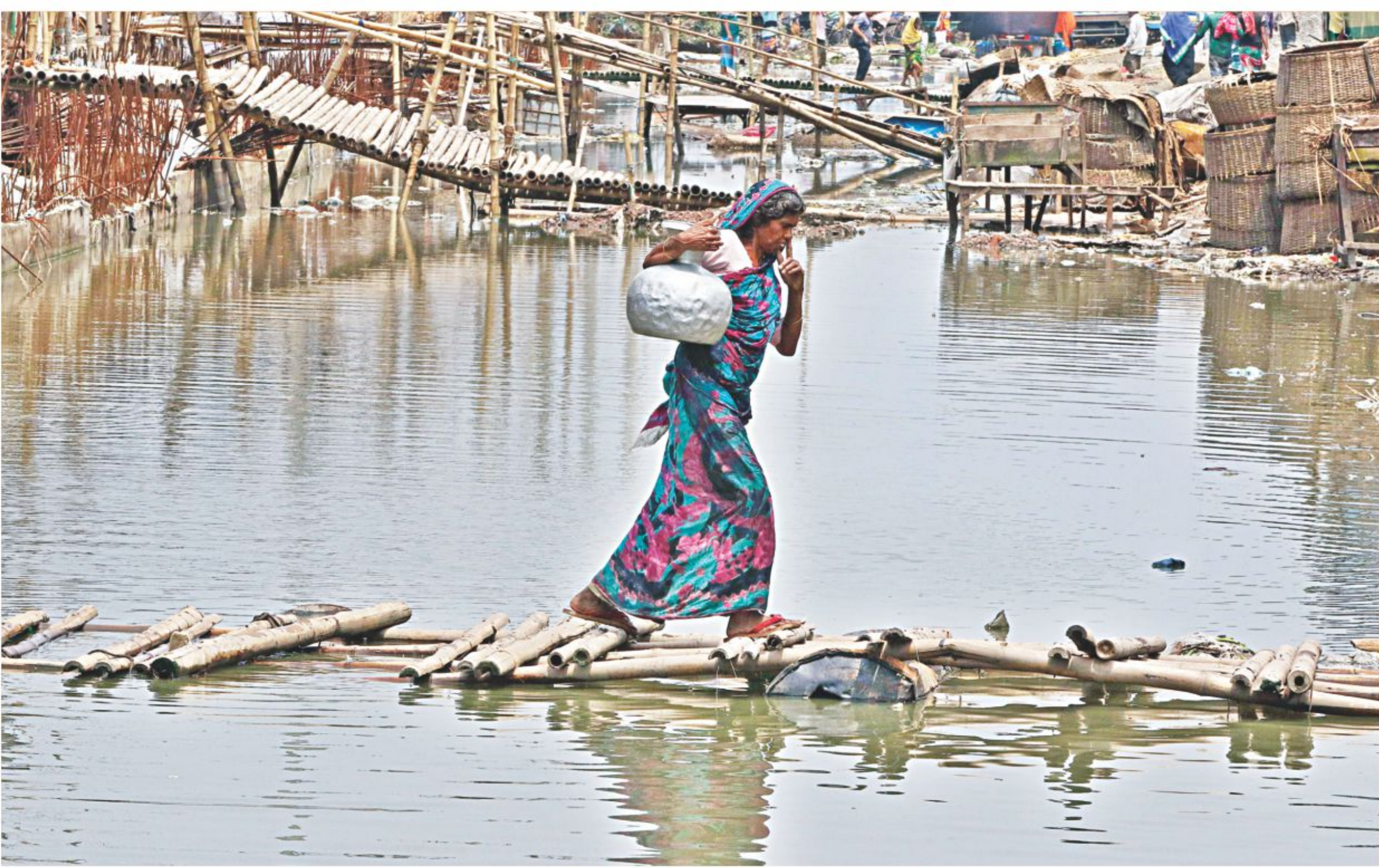
A woman with a pitcher crosses a makeshift bamboo-made bridge on the Dhaka-Chittagong highway. Dhaka South City Corporation is building a drain and pavements in Kutubkhali area of Jatrabari. But the contractor there has made such a trench that locals had to build their bridge with barrels attached to it so that it floated on the stagnant water.
