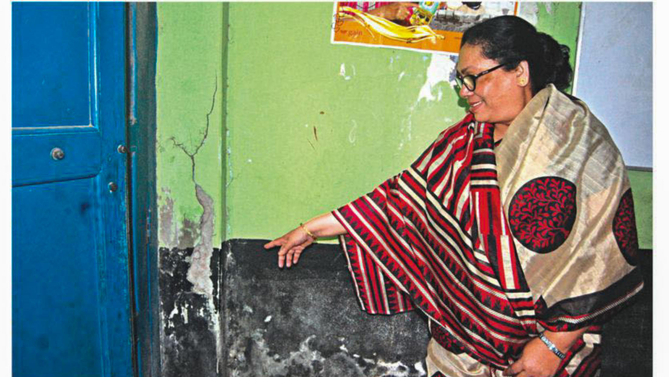
Kazi Shirin Sultana, a head teacher of the school, shows a crack that developed on a column of the wall inside the school building.
