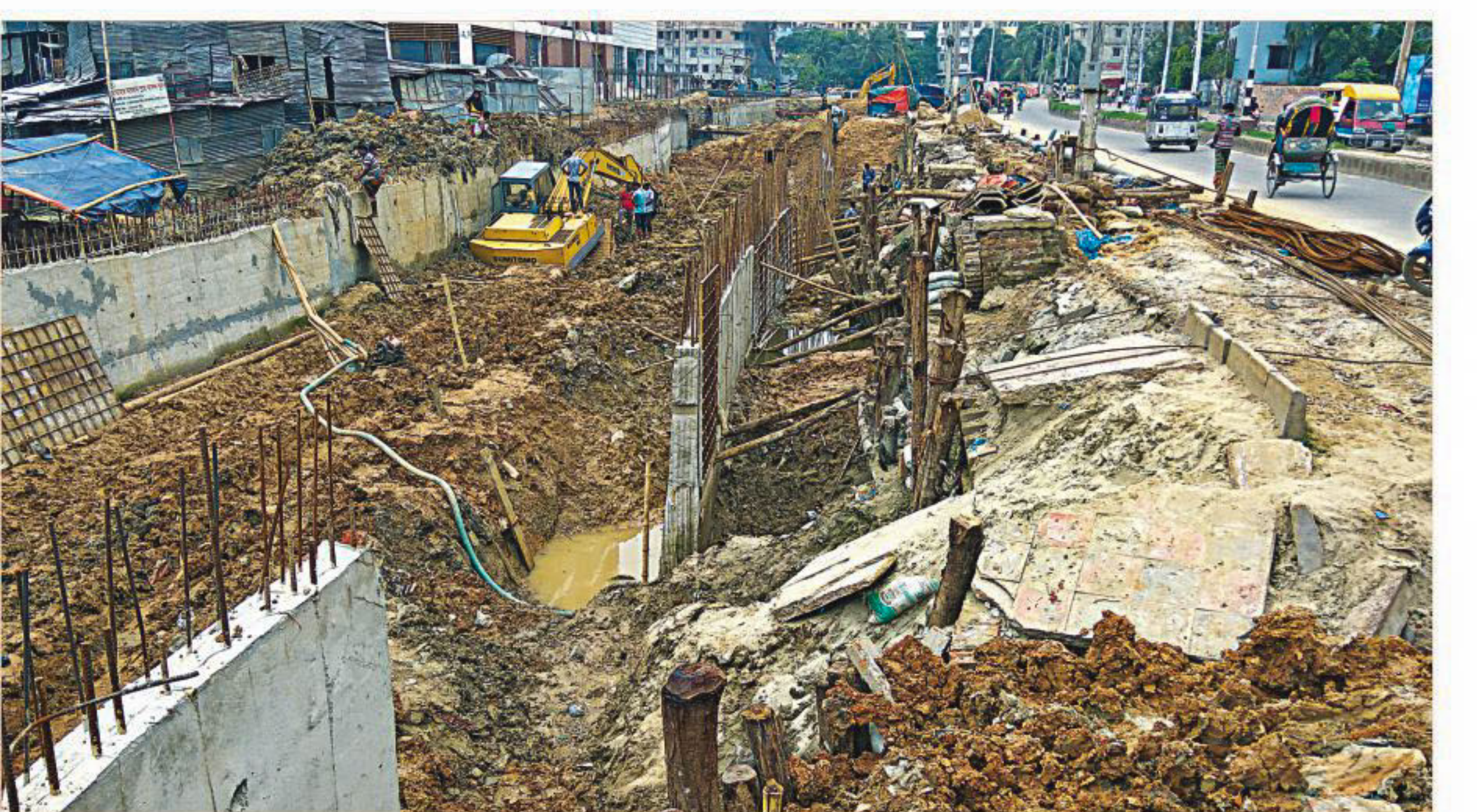
Dhaka Water Supply and Sewerage Authority (Wasa) conducting renovation works in the West Agargaon canal, which include dredging and building of concrete canal linings. After implementation, the canal will drain more waste water and help prevent waterlogging in the area. But the way the works are being done involves risks as Wasa has not built a fence along the road to prevent accidents and erosion of the road, particularly during rains. The photo was taken yesterday. PHOTO: RASHED SHUMON
