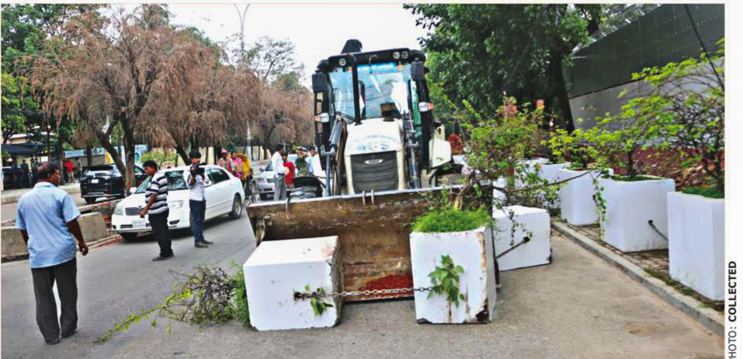
A bulldozer of Dhaka North City Corporation (DNCC) removes concrete planter blocks from the footpath in front of the boundary wall of Australian high commission on northern Gulshan Avenue in the capital yesterday following agreement reached between the DNCC and embassy officials. In a bid to ease pedestrian movement, the DNCC has already removed similar obstructive materials placed alongside sidewalks around the boundary walls of American embassy, Canadian high commission and mission offices of Italy, Russia, Saudi Arabia and Pakistan.
