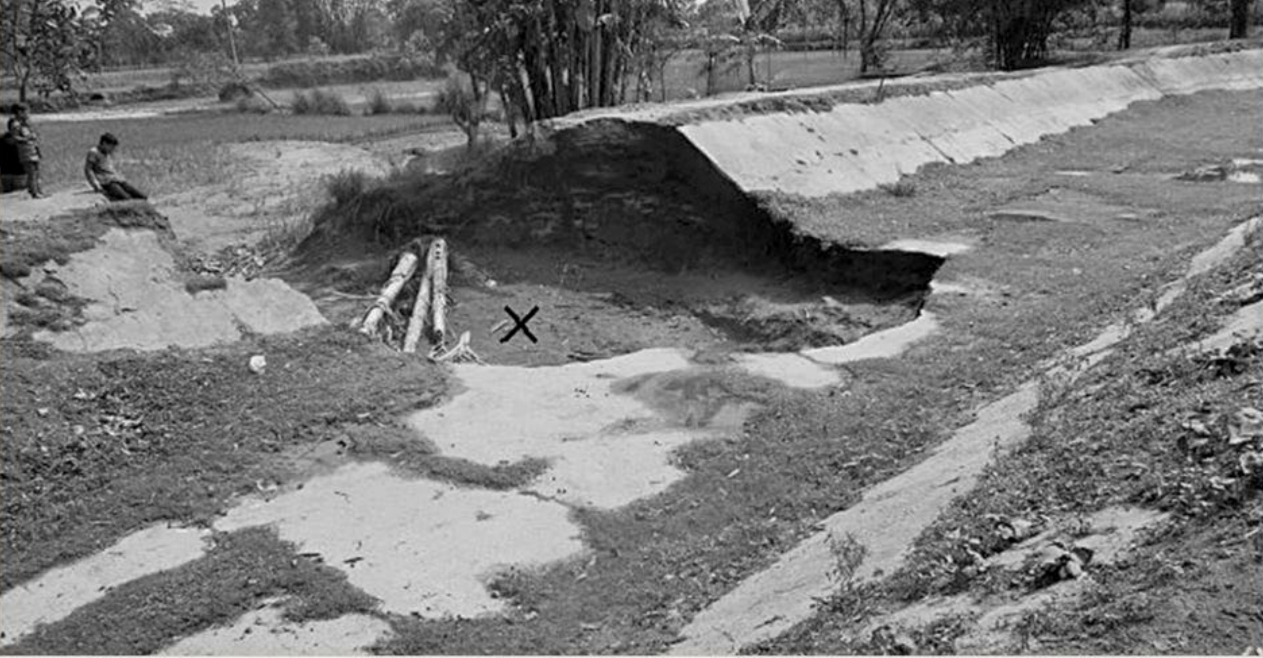
A secondary canal of Teesta Irrigation Project remains dry as the authorities had to close the sluice gates of a regulator in the upstream following breach of the canal embankment on April 12, after unscrupulous people set plastic pipes to illegally draw water at Putimari Kacharipara village in Nilphamari's Kishoreganj upazila.
