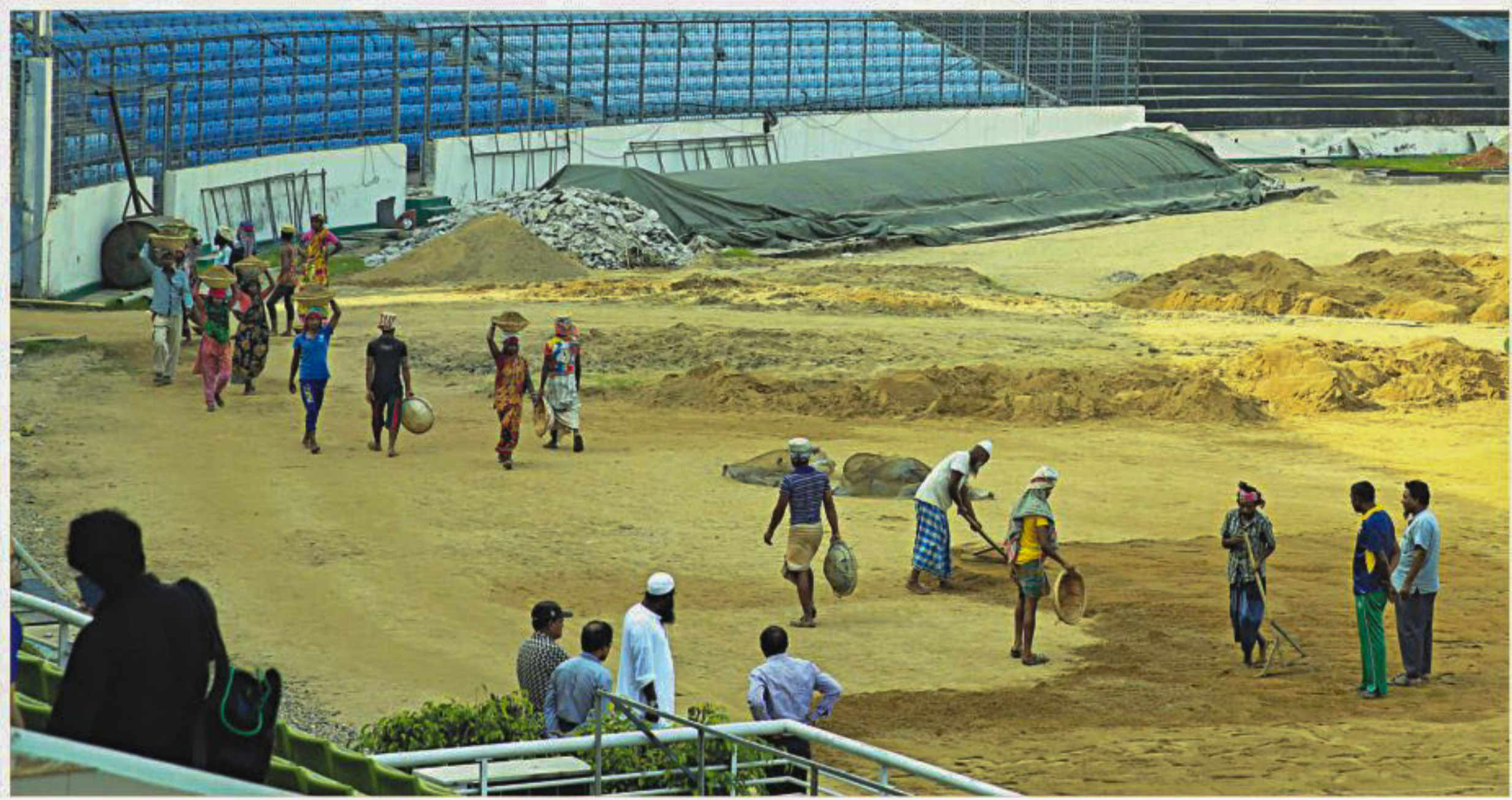
Bangladesh's home of cricket, the Sher-e-Bangla National Stadium in Mirpur, has hosted a glut of matches without a break, causing damage to its turf and most notably the world-class drainage system. This picture, taken recently, shows extensive renovation works in progress, which has bred uncertainty over whether the stadium can host matches during Pakistan's tour of Bangladesh in July-August.
