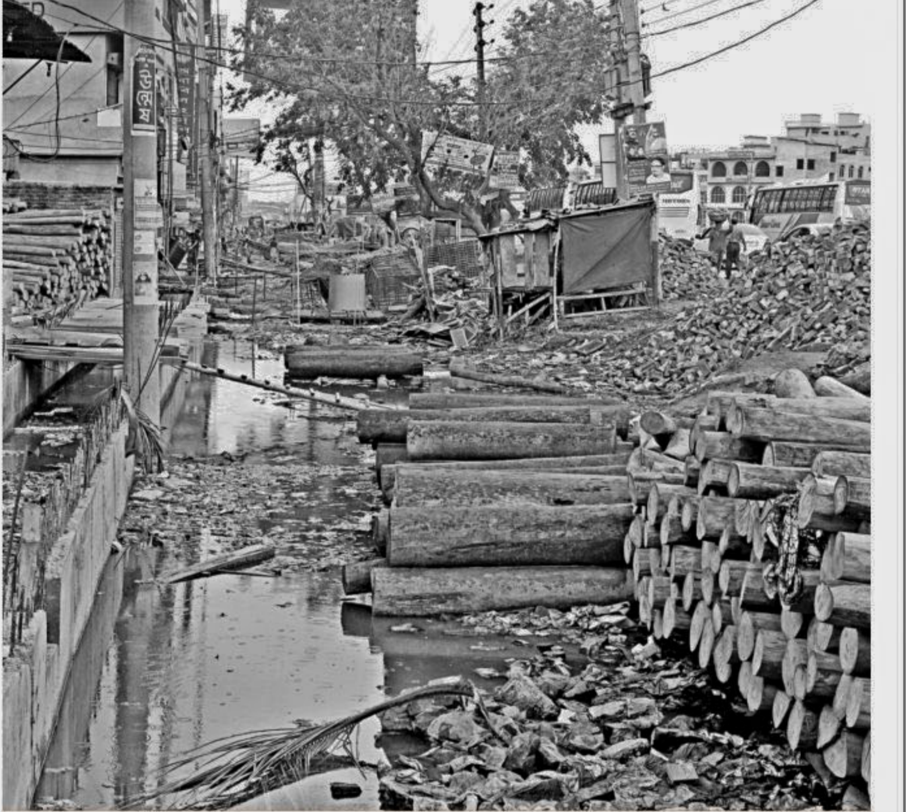
Logs and brick chips are left on a road next to the Dhaka-Chittagong highway in the capital's Shanir Akhra area blocking pedestrians' movement. Also, water littered with garbage remains stagnant on the side of the road due to an ongoing work for the development of the area's drainage system. The work has been continuing for almost a year, prolonging public suffering. The photo was taken yesterday.
