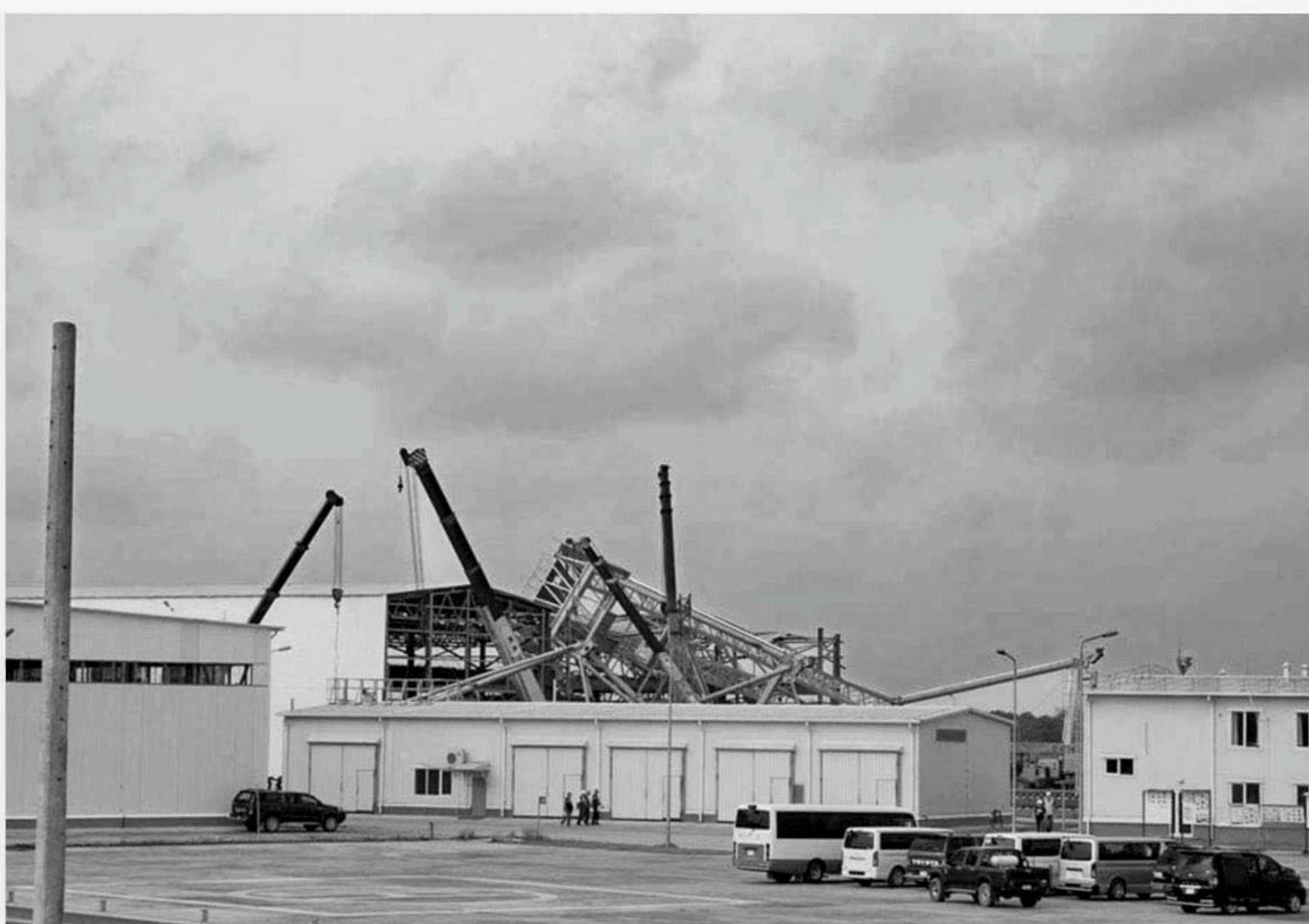
A crane of Roopur Nuclear Power Plant in Ishwardi upazila of Pabna fell down during a storm on Wednesday night, causing damage to this under-construction site of the plant.
